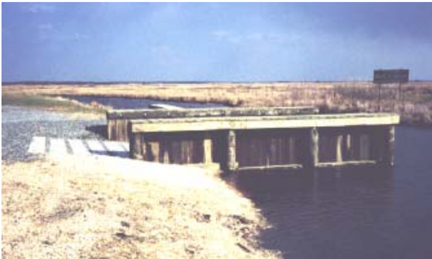
Photo 11A: Geocell material provides paddlers with a “soft” launching alternative to a traditional boat launch
