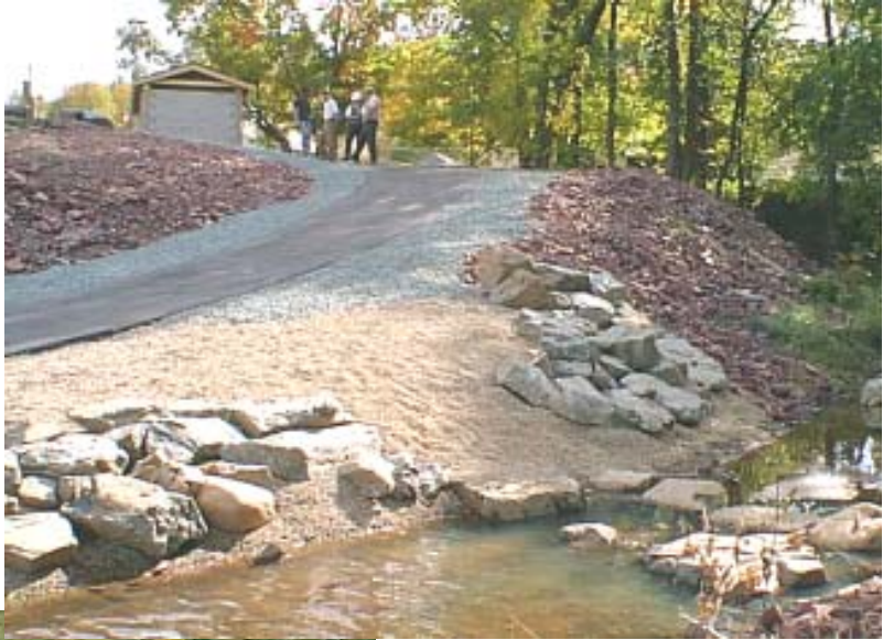
Photo 10B, 10C: Asphalt path leading to launch area below Little Quinnessec Falls Dam
