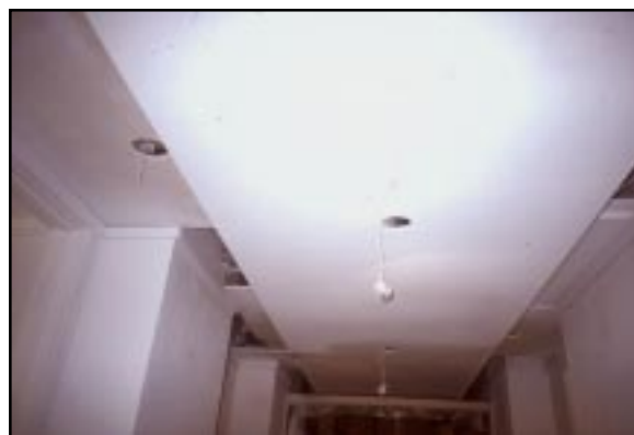
A partial ceiling can cover new systems in a corridor without obscuring existing historic features.
