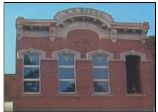
After rehabilitation, the new windows have a three-part configuration that is inappropriate to the historic style of the building.
