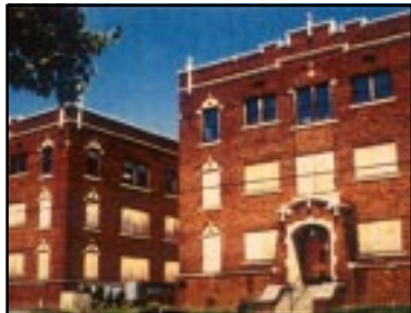
Prior to rehabilitation showing one-over-one sash. Similar sash is concealed by plywood covers on the first and second floors.
