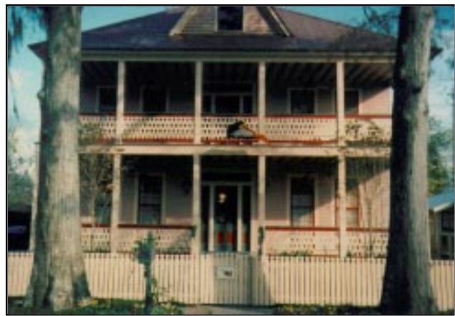
After rehabilitation - inappropriate replacement balustrade.
