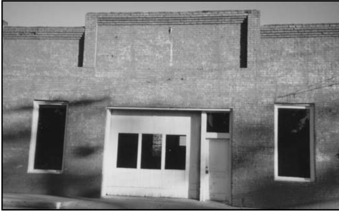
Before the work began, the original 1930 garage door opening had an operable garage door and a pedestrian door surmounted by a glazed transom installed as infill.
