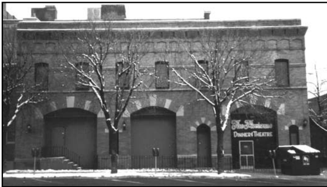
The south elevation of the 1903 firehouse is dominated by three large garage door openings. This photo was taken just prior to rehab and shows the existing infill treatments.
