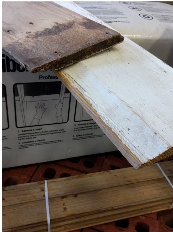
Figure 3. Selection of new and reclaimed materials procured for this project, with evidence of existing mold and coatings on the two styles of reclaimed siding.
