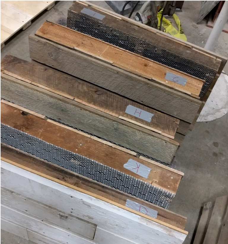
Figure 6. Walls D, F, G, H, and K prepared for plaster and stucco application.
