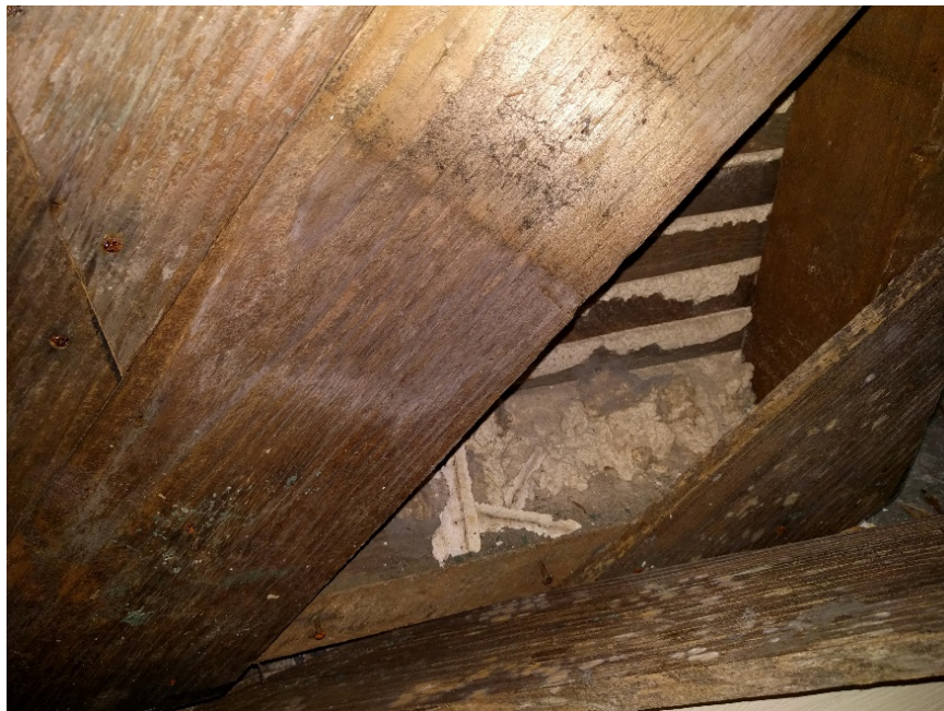
Figure 44. Photograph of Wall D cavity after drying, showing heavy contamination.
