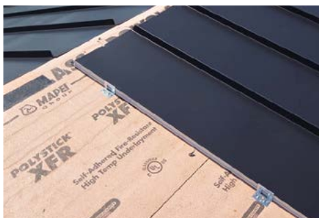
Figure 17: Even a Class-A roof assembly can admit embers if gaps are left unsealed, so fire-rating and ember-resistance requirements must be paired. Open ends of clay tile roofing (left) should be plugged. Metal roof assemblies (right) should interrupt rapid heat transfer to combustible substrates, such as by using a fire-resistant, high-temperature underlayment as shown here. Photos: (left) NPS; (right) Local Roofer, Inc.
