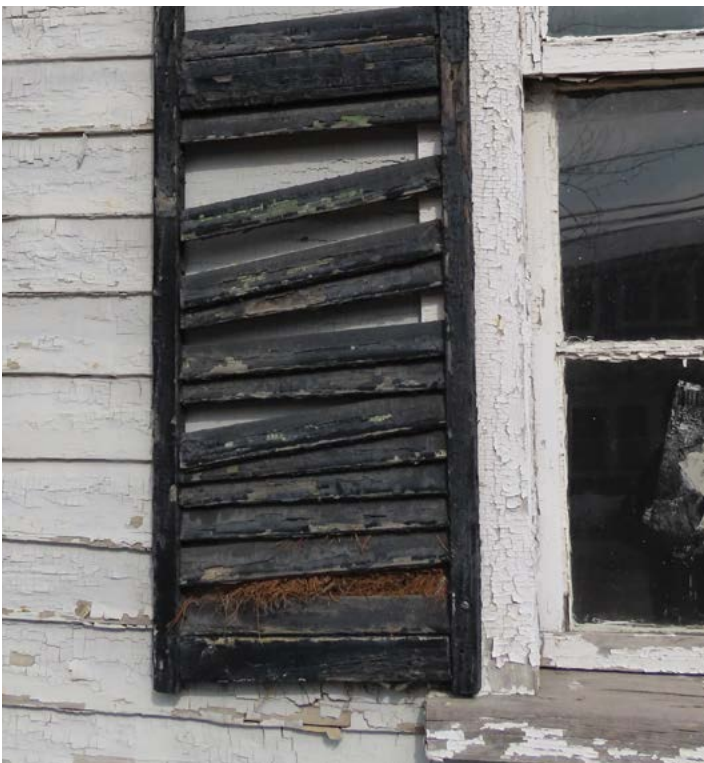
Figure 25: Deferred maintenance such as peeling paint, cracked cladding, failed shutters, and nesting debris increases the risk of ignition and loss from wildfires. Photo: NPS
