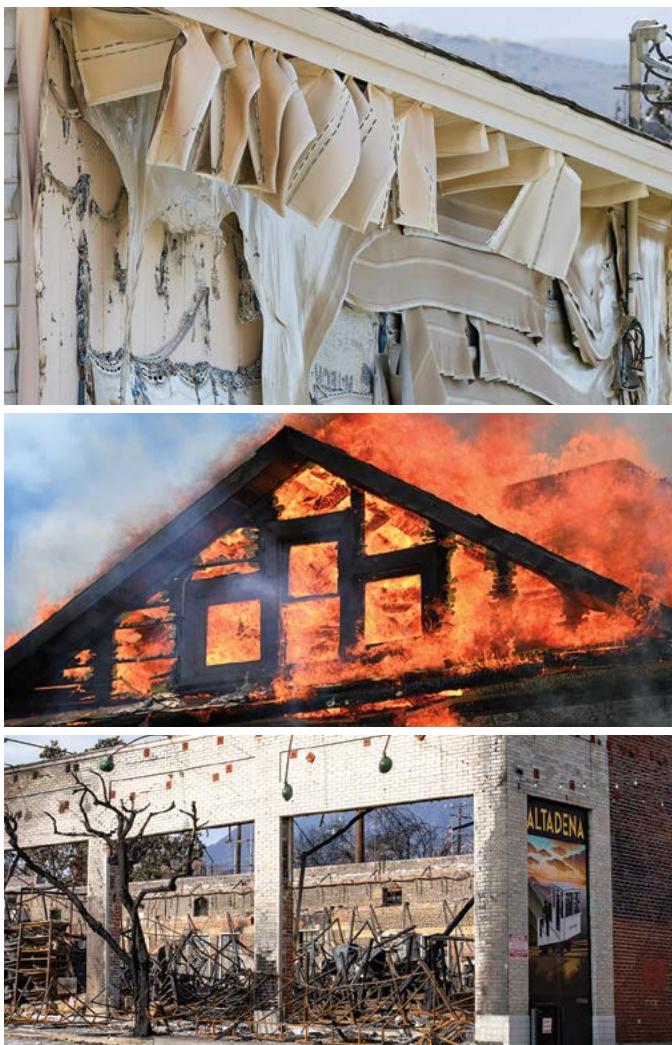
Figure 6: Heat-vulnerable materials like vinyl soften and deform under low heat (top); combustible materials like wood ignite and burn even more quickly when dry (middle); noncombustible materials like masonry resist ignition but can still fail under prolonged extreme heat (bottom). Photos: (top) Fred Greaves / Reuters; (others) Shutterstock
