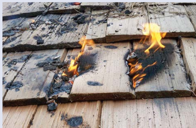
Figure 9: Untreated wood roofs are highly vulnerable to ignition, as flying embers easily lodge in the rough texture and joints. Adaptive treatment options for wood roofing should be carefully considered. Photo: University of Nevada, Reno Extension
