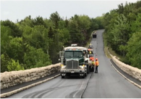
Typical mill and overlay pavement preservation treatment at Acadia National Park. (Photo credit: NPS)
