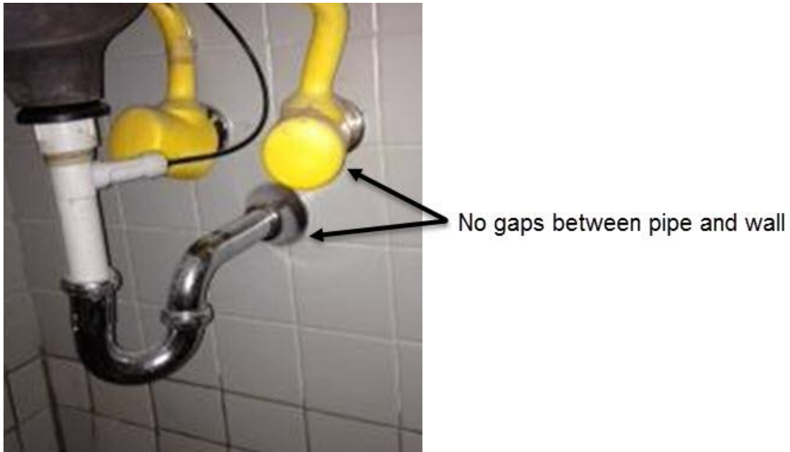
Figure 16: Evaluate service entry points. Here plumbing entrance points are sealed using a commercial flange that is sealed to the wall tile using caulk. Figure credit: NPS Figure.
