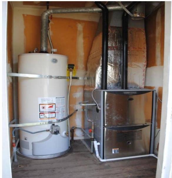
Figure 17: Evaluate utilities for potential entry points, which are commonly found behind the hot water heater or furnace. Also check for nesting material underneath or behind these appliances. Figure credit: Bruce Badzik.
