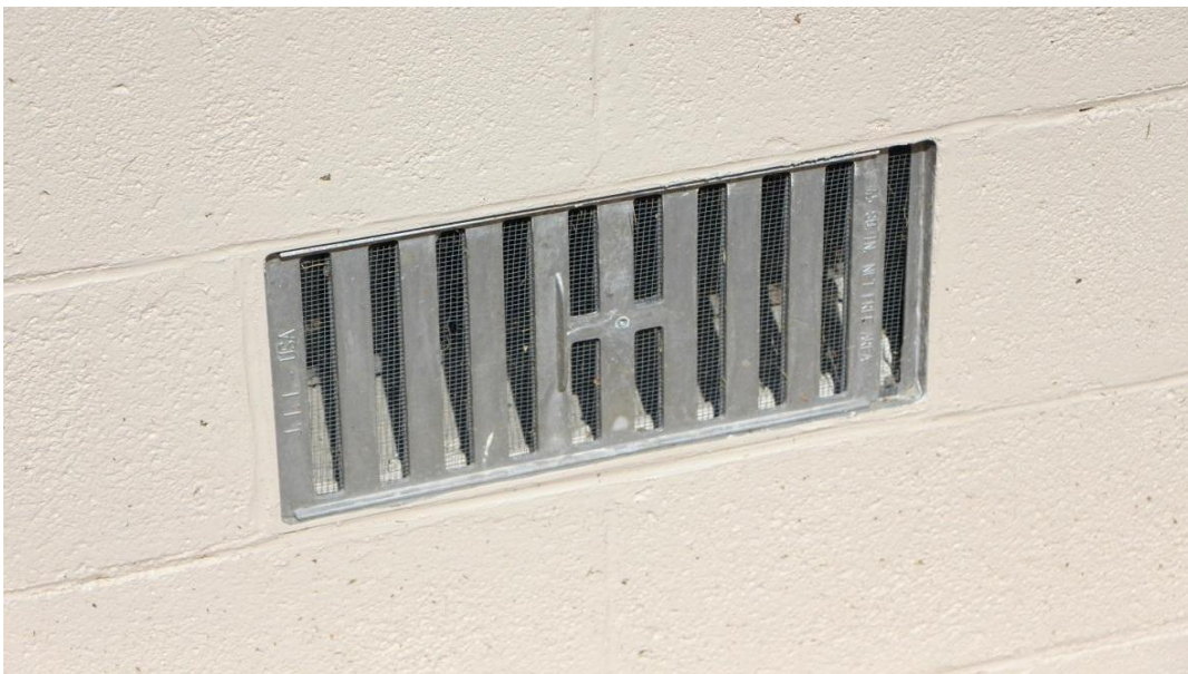
Figure 7: This crawl space vent is properly screened with \frac{1}{4} " hardware cloth (visible behind the metal bars). Figure credit: NPS Figure.
