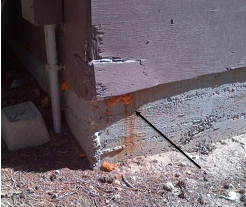
Figure 30: Expanding foam can be used to fill gaps. This foam must be trimmed and painted once dry to protect it from breaking down or becoming brittle in the sun's UV rays. Figure credit: NPS Figure.
