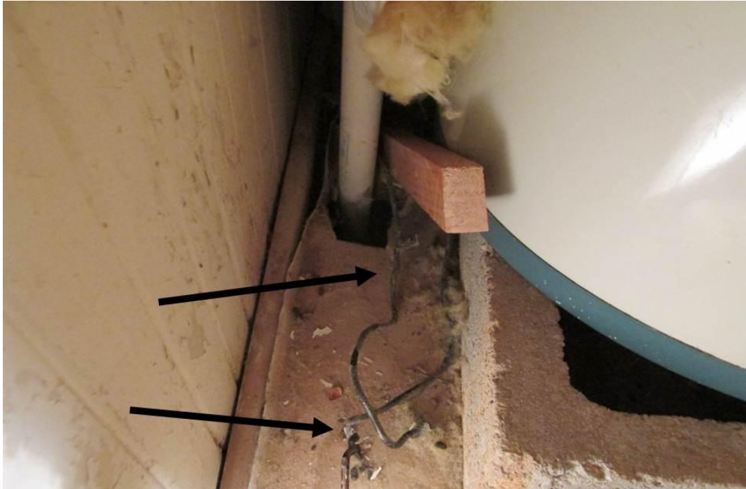
Figure 20: Wire damage from packrats. Figure credit: Charles Conner.
