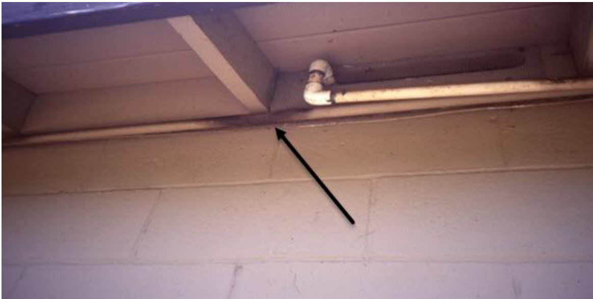
Figure 21: Grease marks from a Roof rat ( Rattus rattus ). Figure credit: NPS Figure.
