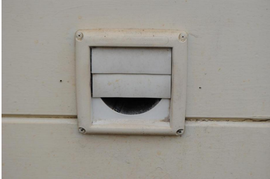
Figure 5: The lower exhaust flap on this dryer vent is missing and provides rodents access to the building interior. A new rodent proof flap needs to be installed with ¼ inch hardware cloth to exclude rodents. The vent must also be periodically cleaned to prevent lint build up. Figure credit: NPS Figure.
