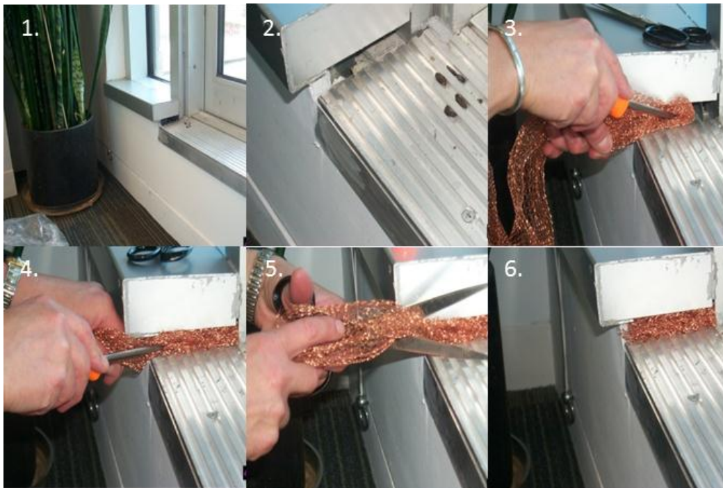
Figure 38: Steps for installing copper mesh to exclude rodents: fecal pellets (droppings) were detected, area was cleaned with bleach, and snap traps were set. Stuf-Fit® copper mesh was installed to eliminate rodent access point. Figure credit: NPS Figure.
