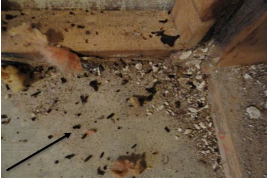
Figure 18: Rodent feces (droppings) confirm rodent activity in this wall void. Figure credit: Carol DiSalvo.
