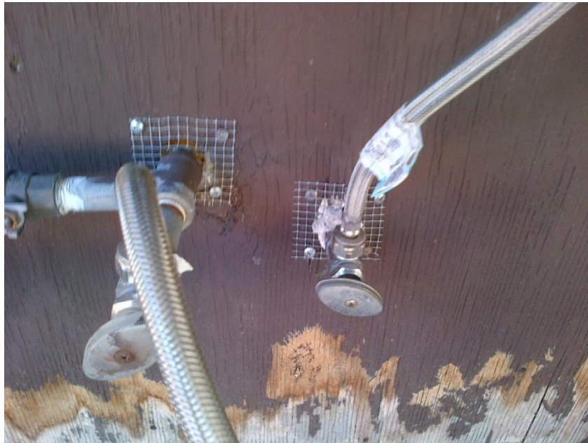
Figure 29: Methods to fill gaps can include caulk and ¼ inch hardware cloth fastened with a staple gun or screws. Figure credit: NPS Figure.
