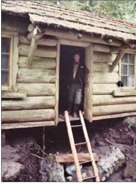
Above: A channel of the Carbon River carried away the ground beneath the historic Ipsut Creek Cabin.
