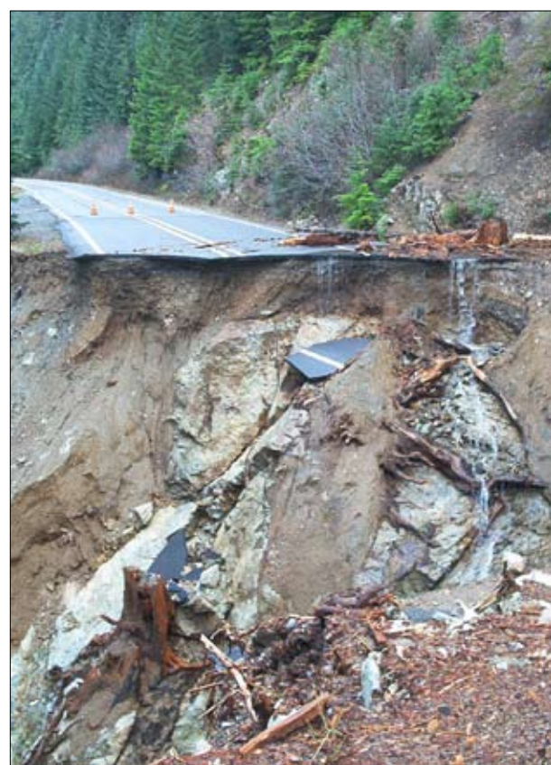
One of four washouts on Highway 123, between Ohanapecosh and White River.
