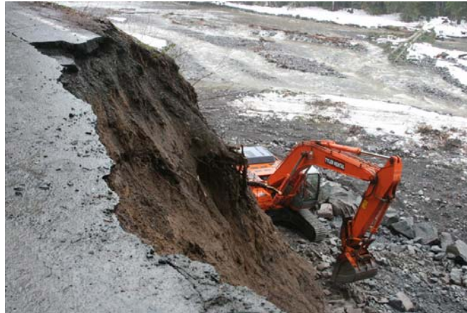
Work continues at Milepost 5.2 on the Nisqually Road. The road will reopen to the public in May.
