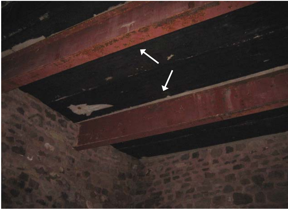
Figure 93. Steel I- beams (at arrows) supporting the modern concrete floor slab at the south end of the connecting shed, September 2007.
