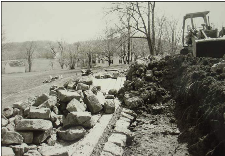
Figure 72. Wall restoration at the east head race, on the west side of Route 345, spring 1984.
