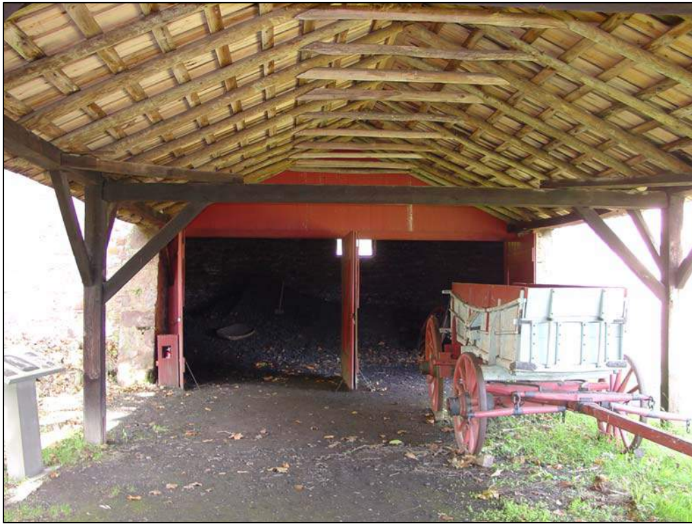
Figure 89. Interior view of the connecting shed, looking north towards the charcoal house, September 2006.
