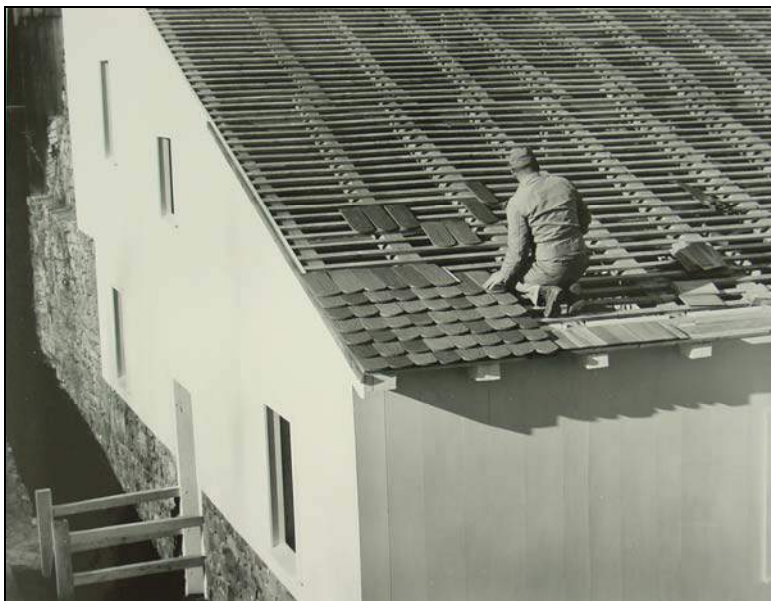
Figure 62. Installing tile shingles on the south slope of the cast house roof, November 17, 1964.
