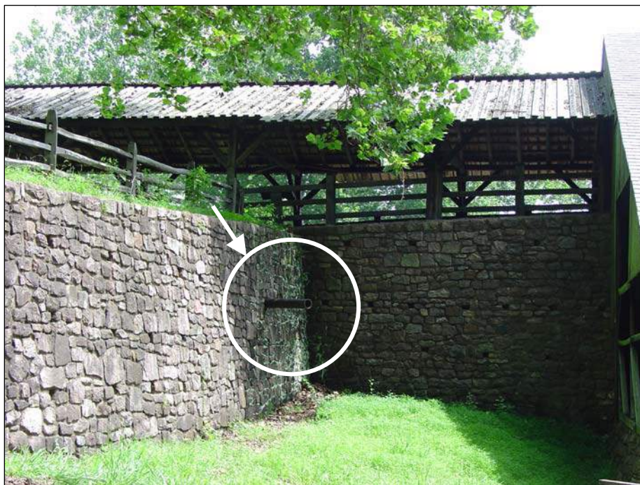
Figure 105. Truncated pipe (at arrow) that conveyed water from the east head race to a wooden flume (now missing) north of the water wheel, July 2006.
