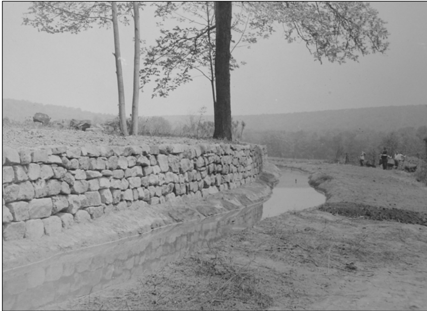
Figure 36. View of the restored retaining wall of the east head race, looking east, May 1939.
