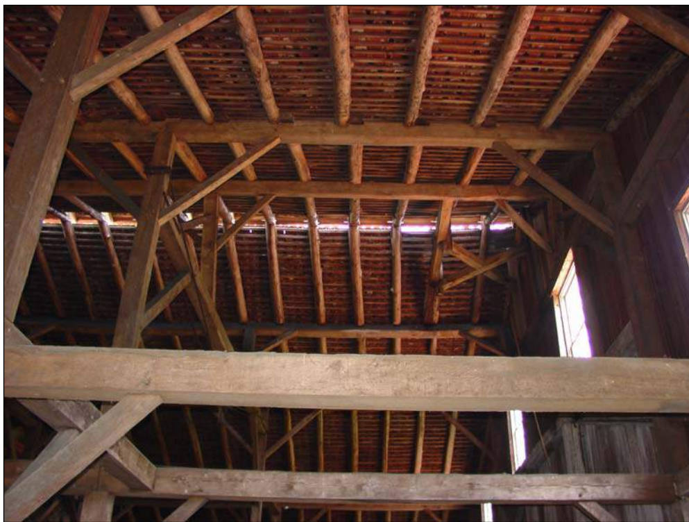
Figure 119. Detail of interior roof framing of the cast house at main ridge, July 2006.
