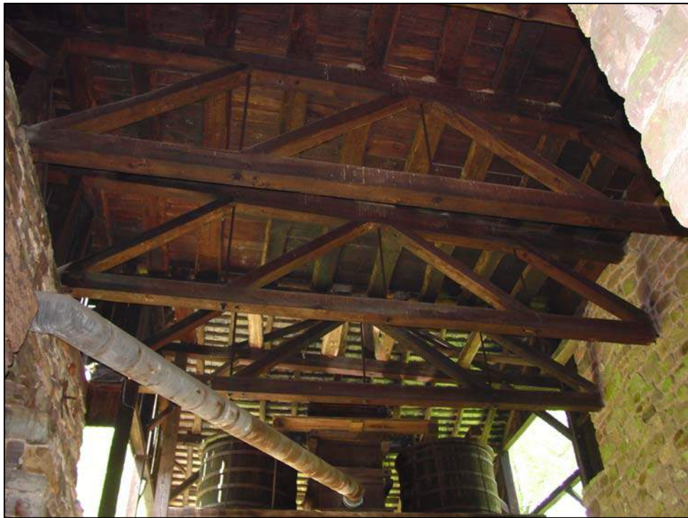
Figure 92. View of floor framing of the enclosed bridge house and tunnel-head vestibule, looking west, July 2006.
