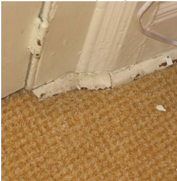
Fig. 65 : Wood baseboard, bead molding, and carpet at the Officer in Charge Quarters.
