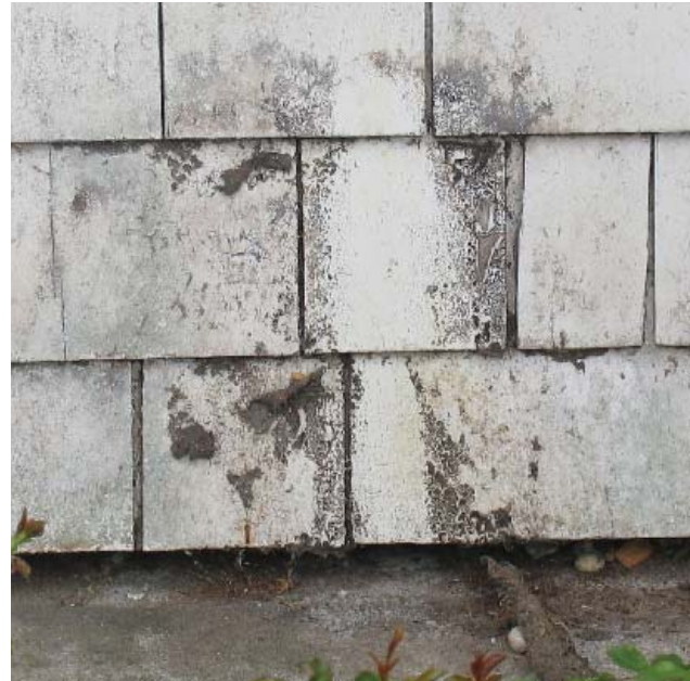
Fig. 50: Shingle soiling and deterioration at the Main Boathouse.
