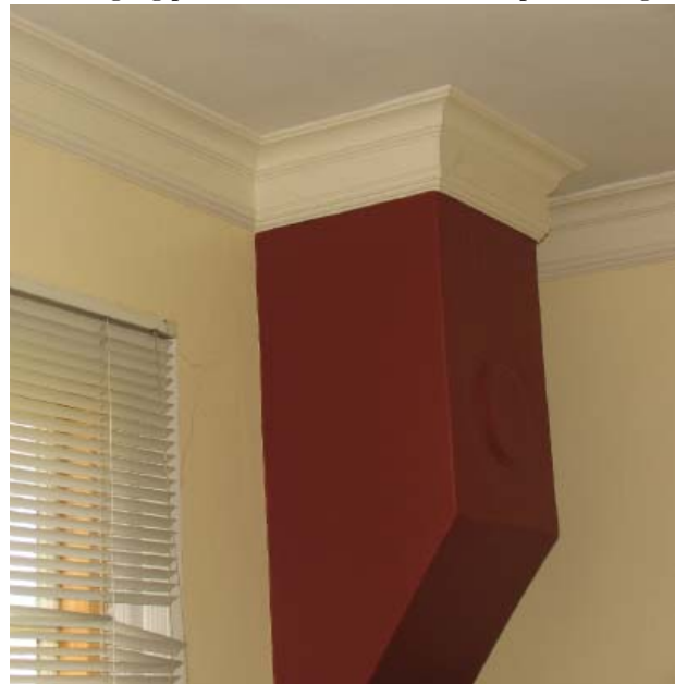
Fig. 74 : Flue and flue cover at the Officer in Charge Quarters, remnant of earlier stove heating system.
