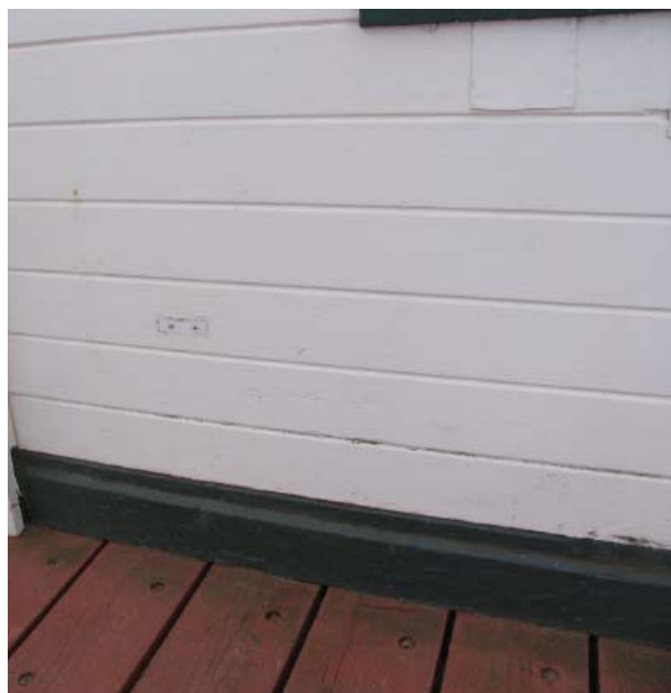
Fig. 44: Inappropriate patching on clapboard wall at the Buoy Shack..
