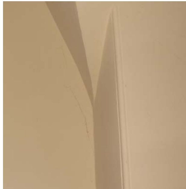
Fig. 60 :Flat plaster wall and corner bead at the interior of the Officer in Charge Quarters.
