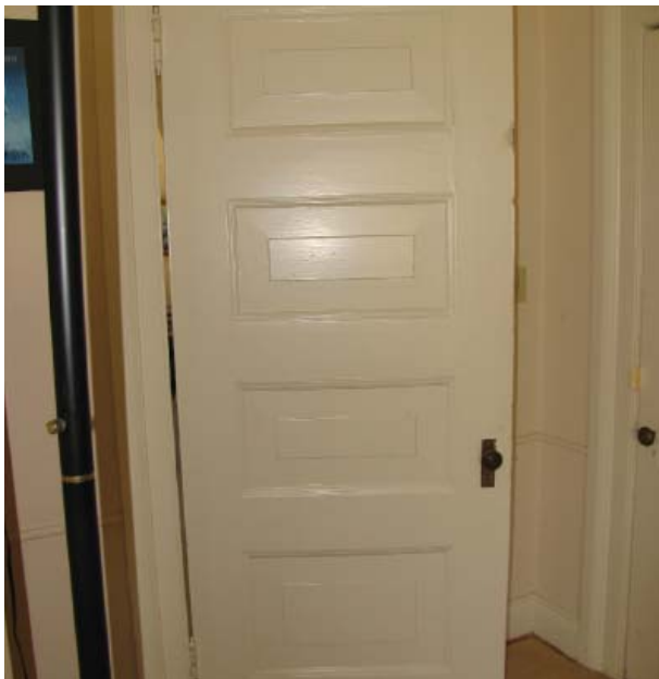
Fig. 67 : Most of the doors appear to be in good condition, with only minor repairs needed.
