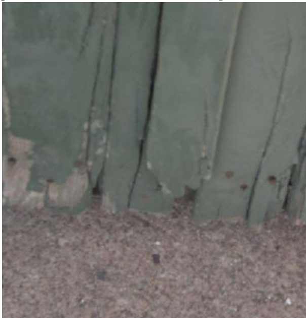
Fig. 45: Mechanical deterioration of doors of the Shop & Garage associated with cross-grain dragging.
