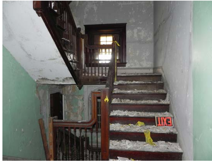
Stairs leading to the third floor of Building 6. Photo taken September 2014. NPS PHOTO
