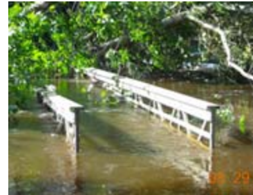
The McDade footbridge went under as Hurricane Irene swelled the Raymondskill.
