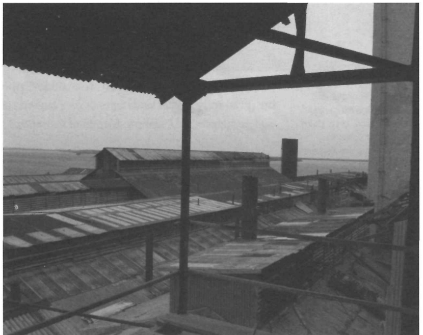
FIGURE 2 Looking out over the rusting corrugated metal roofs of the now derelict Central Aguirre mill. (Sam Sweitz, photographer).
