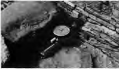
This dial gauge installation produced the data in the line chart. The gauge is mounted on top of a wall on one side of the crack. A metal plate is attached to the taller back wall. The spring-loaded spindle of the gauge rests on the metal plate, but is not attached to it. As crack width changes, the spindle moves and changes the position of the gauge hands.
