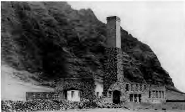
1860s mill at Kualoa, O'ahu. Wilder Sugar operation ran from circa 1864-1870. Photo circa 1920. The stone walls have further deteriorated. Photo courtesy Hawaiian Mission Children's Society (HMCS).
