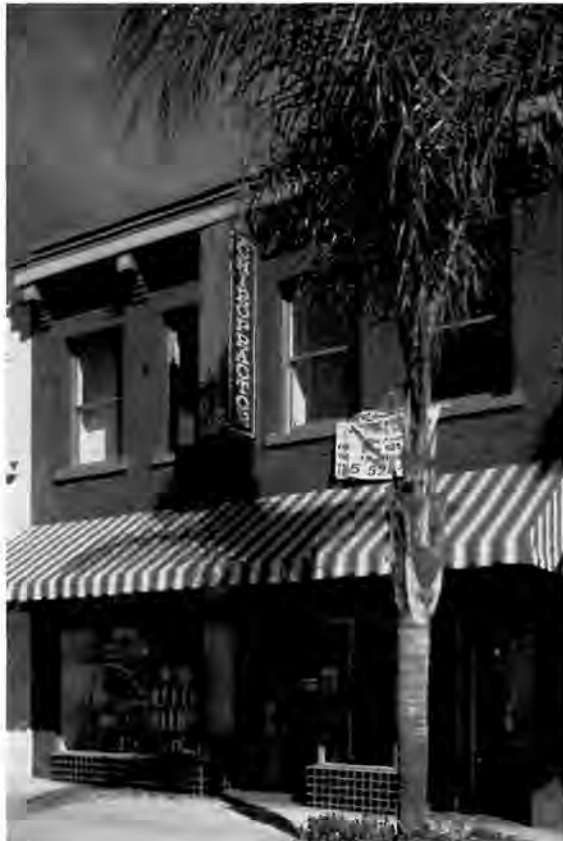
The Fillmore Commercial Buildings in Los Angeles County, California were seismically retrofitted without altering the brick facades. Photo courtesy Historic Preservation Partners for Earthquake Response.
