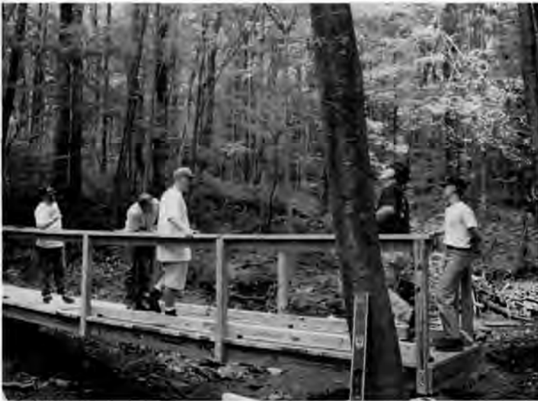
A number of community partnerships have helped develop interpretive trails on the battlefield. In June 1996, local Eagle Scouts built a footbridge on the trail to Camp Garnett. Photo courtesy RMBF.
