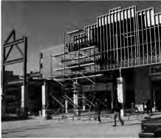
Bala Cynwyd Shopping Center, Bala Cynwyd, Pennsylvania, built ca. 1960, receiving a new Dryvit facade. Photo by Rebecca Shiffer, 1991.
