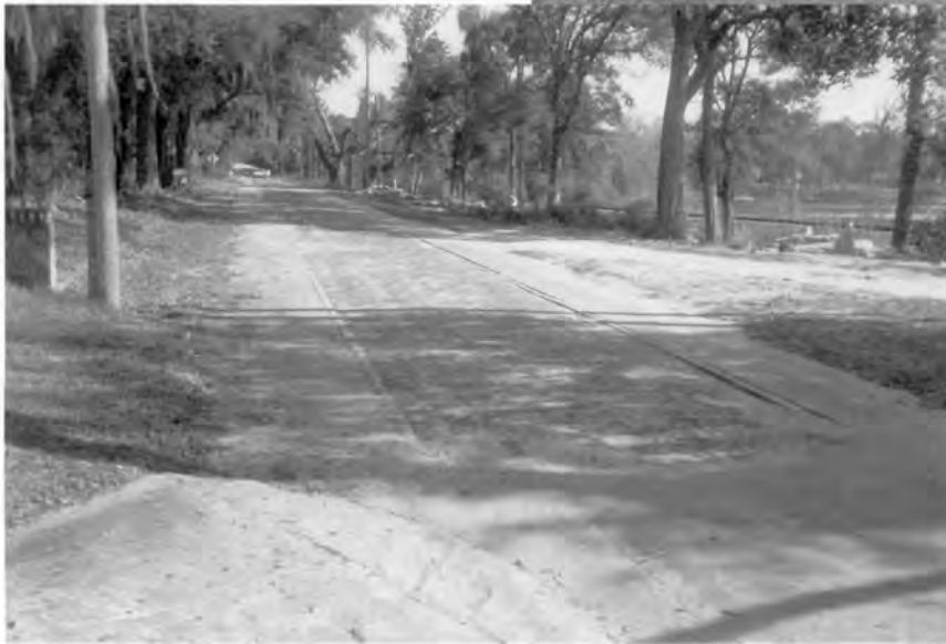
Completed in 1921, Florida State Road No. 1, Santa Rosa County, FL, was the first paved highway in West Florida. This six-mile long, 24' wide brick section of the road was planned as part of the Old Spanish Trail from Jacksonville, Florida, to the Pacific Ocean. Ironically, in 1977, bricks removed from a half-mile long section at the eastern end of this original road segment were used to construct a memorial sidewalk commemorating the historic Old Spanish Trail. Photo by Barbara E. Mattick, Bureau of Historic Preservation.
