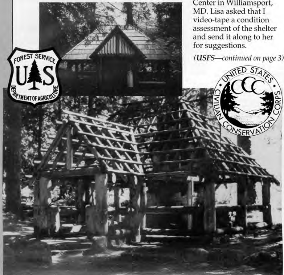
Tollgate Shelter with roofing removed (below) and after restoration (above). Photos by the author.
