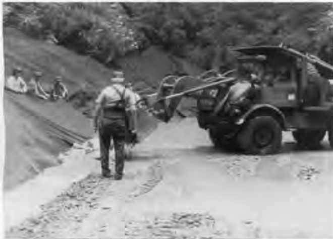
Fig. 2. Primary panel of filter fabric being stretched out. Base of the fabric is anchored in the channel seen in the lower left-hand corner of the photo. Rocks are being placed over the fabric to firmly anchor it in the channel.
