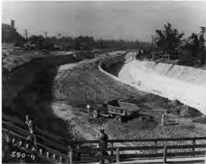
Construction of the Arroyo Seco Parkway, 1939. Like the Bronx River Parkway, the Arroyo Seco Parkway (Pasadena Freeway) paralleled the river course and provided open space for liesure, recreation, and aesthetic enjoyment. Photo courtesy Caltrans.
