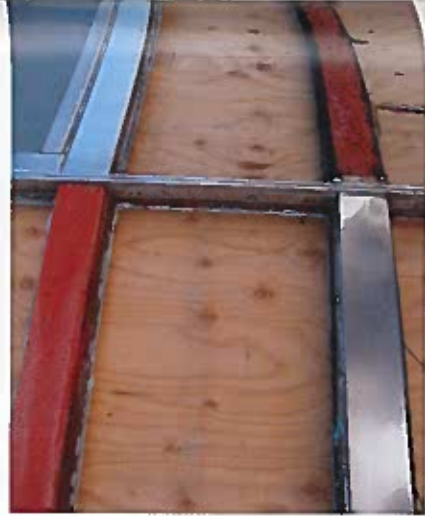
In the old window system, a thin layer of stainless steel failed to protect the plain steel frame.
