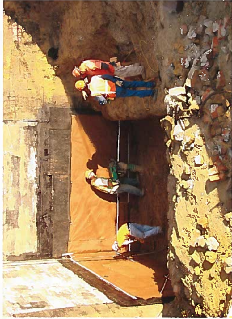
A deep pit reveals the back wall of the east bleacher.
