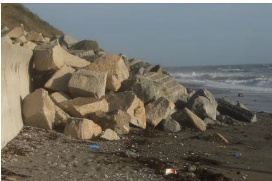
Poorly constructed riprap
