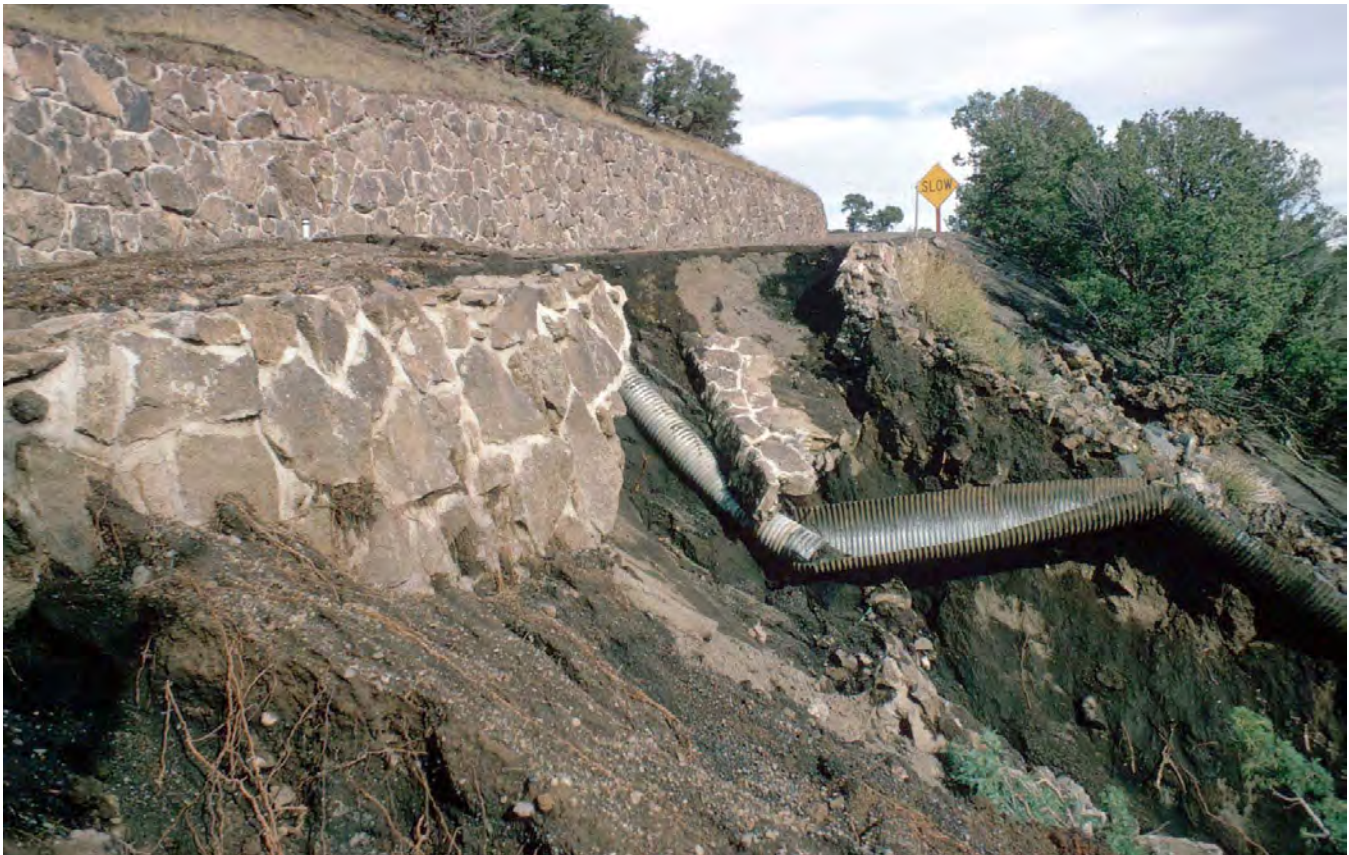
Figure 28. Photograph of storm-related damage along Volcano Road. Erosion on Capulin Volcano is primarily associated with Volcano Road. Culverts provide narrow paths for storm-water runoff, creating erosion channels and gullies down the sides of the mountain. National Park Service photograph (date unknown).
