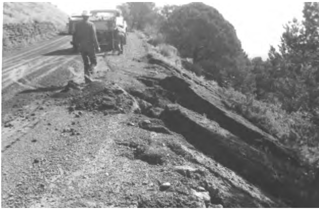
Figure 30. Photograph of erosion along Volcano Road. In spring 1967 Volcano Road was closed while monument personnel assessed damages and made repairs. In 2012, a Federal Highways Administration project remediated some areas of severe erosion along the road. National Park Service photograph from Bennetts et al. (2012, figure 4.5.1-7).
