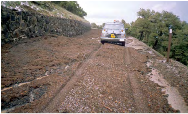
Figure 32. Photograph of a debris flow on Volcano Road. Slope movements are a common type of geologic hazard—a natural or human-caused condition that may impact park resources, infrastructure, or visitor safety. Debris flows have impacted Volcano Road, causing road closures and trapping vehicles above an affected road section. National Park Service photograph (date unknown).
