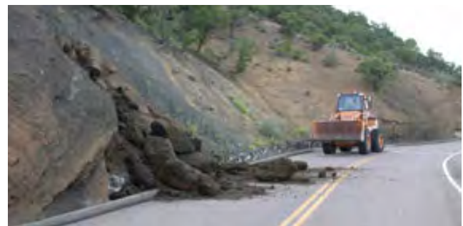
Figure 31. Photograph of a cinder slide on Volcano Road. Slope movements are ongoing at Capulin Volcano National Monument; the slide shown here took place in 2004. Cinder slides are a particular concern along Volcano Road. Keeping the road clear of cinders is a continuous maintenance activity. National Park Service photograph available at http://www.nps.gov/cavo/naturescience/environmentalfactors.htm (accessed 19 November 2014).
