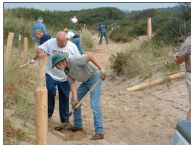
Volunteers install fence at Herring Cove Beach on National Public Lands Day.
