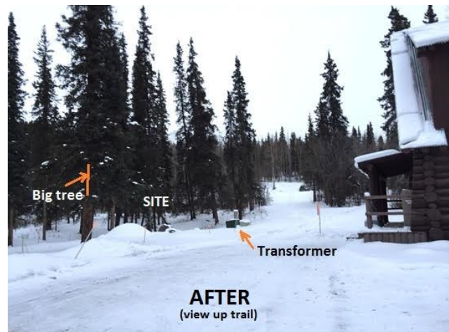
Denali NP&Pres regraded and revegetated site after demolition of obsolete former dispatch center
