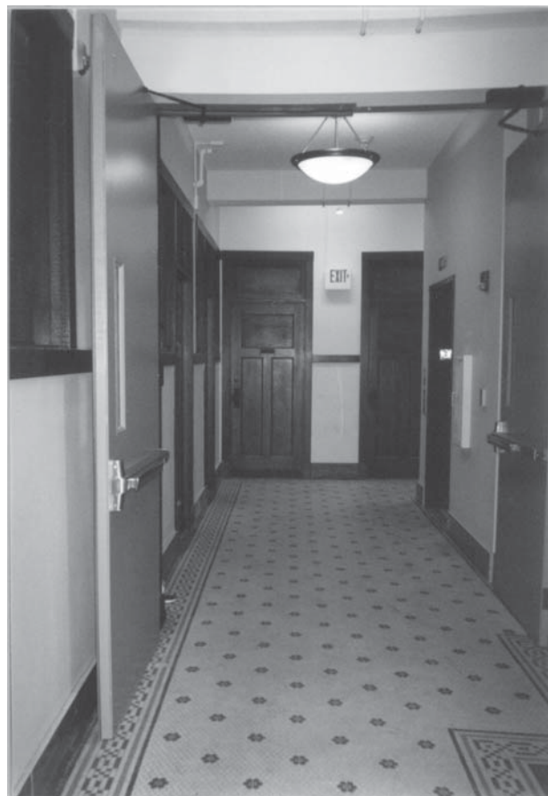
Challenges of fire-rating the interior of the Marsh Place Apartments were met in part through innovative drywall applications that left the historic character of the corridors preserved.
