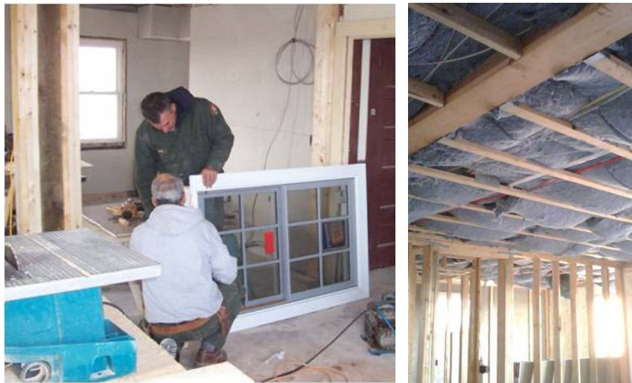
Installation of double pane windows and recycled denim insulation at park ranger stations.
