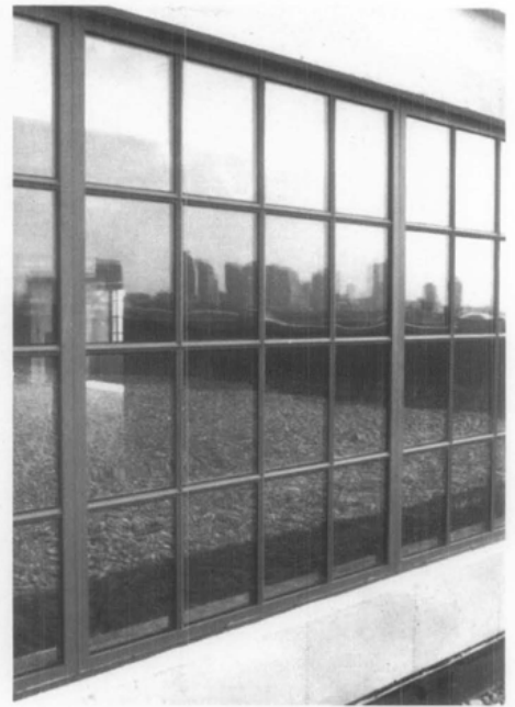
Figure 7. Despite the difficulty encountered with proper glass sizing and spacer alignment in the sealed insulating glass, the end result is an innovative window that is both aesthetically pleasing and closely matches the historic appearance of the original steel design. The slight encroachment of the bronze spacer onto the visible glass area is not readily detectable from general view. Photo: Charles Fisher
