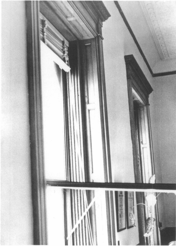
Figure 5. The interior storm window was designed to fit within the existing wooden jamb. The large size of the windows necessitated the use of operable storm panels, intersecting at the historic meeting rail. Here the lower storm panel is in an opened position for cleaning. Photo: Charles E. Fisher
