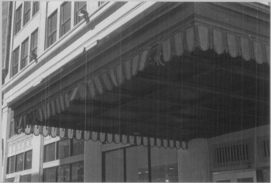
Figure a. Rust, paint failure, open joints, broken glass, or damaged and missing sections are indications that pendant frames are in need of repair.
