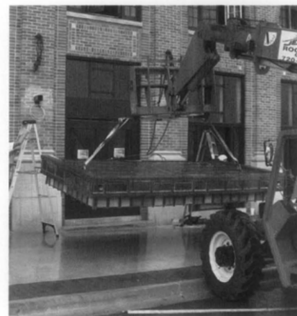
Figure 6. The installation of the new canopy required the use of a Sky Track and a special harness to ensure the protection of the copper frame. Photo courtesy of Thad Jennings, JENCO Roofing & Sheet Metal.
