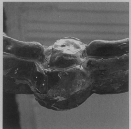
Figure d. Typical deteriorated conditions on pressed, galvanized metal pendants can include broken or missing glass (top); broken or misaligned elements (middle); and rust along the bottom of the pendant frames where water has collected (bottom). These conditions can usually be repaired.
