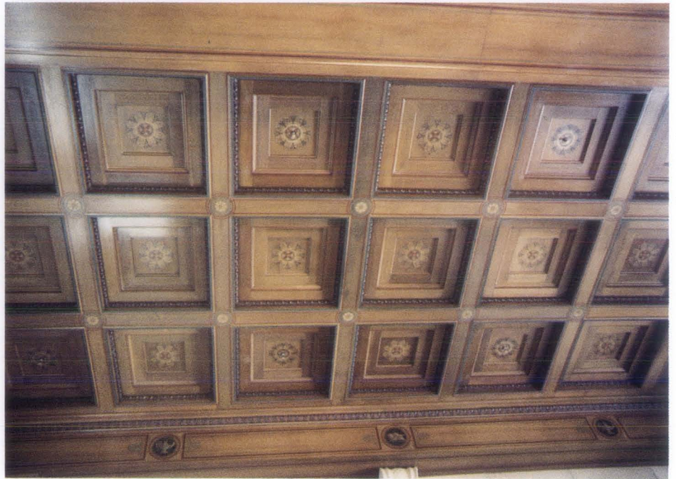
7. Following the work, the difference between the decal replacements and the historic stencilled panels is not discernible from the floor of the Central Search Room. Photo: Dell Corporation.
