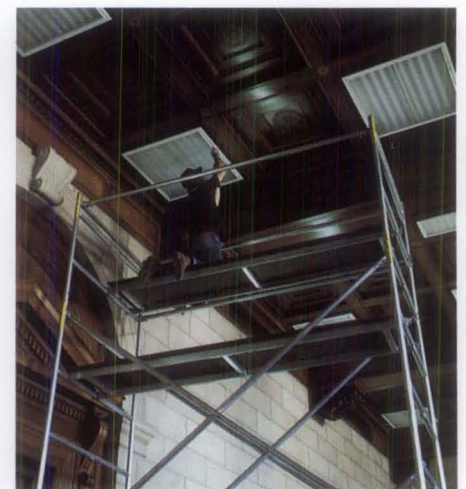
3. The light fixtures were carefully removed to permit installation of a sprinkler system behind the coffered ceiling and to restore the ceiling to its original appearance. It was necessary to reproduce 40 new panels for installation in the coffered ceiling, due to the damage resulting from the 1962 lighting work. Photo: Dell Corporation
