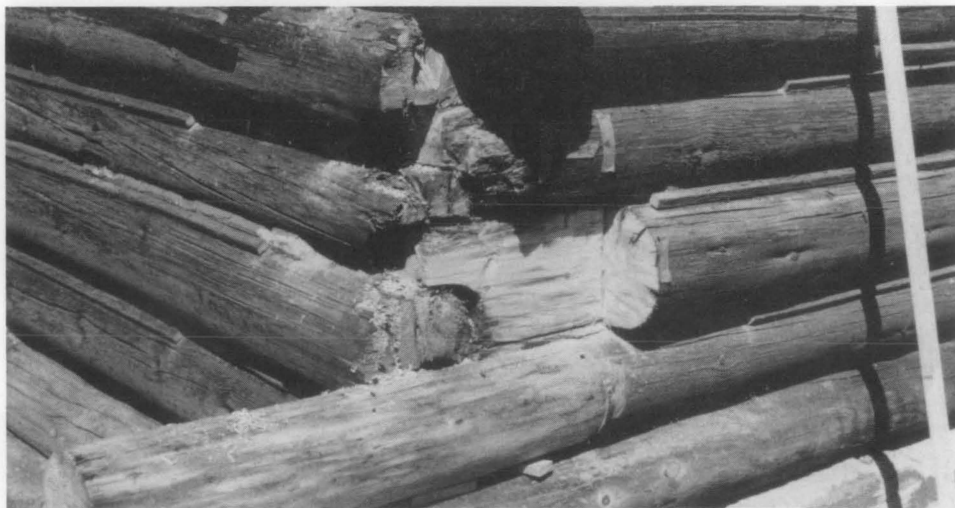
Figure 4. In a few cases, the deterioration had penetrated beyond the center line of the log corners and portions of the wall face were removed. Photo: Harrison Goodall.
