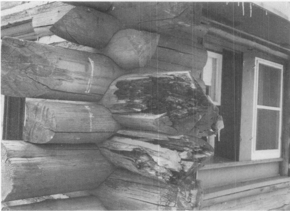
Figure 1. Typical deterioration of log crowns is seen at the Institute Building, adjacent to the Lamar Barn. This is the condition of many of the log crowns at the Lamar Barn prior to the repair and replacement work. Logs are notched at the corners. Photo: Harrison Goodall.
