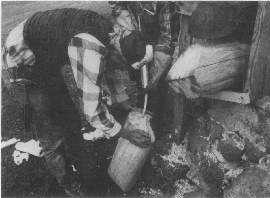
Figure 7. A 12 1/2" long hole was drilled into the new crowns. This hole was filled in the same manner as were the old logs. The crown was then immediately lifted into position and supported by the cribbing framework for several days until the epoxy cured. Photo: Harrison Goodall.
