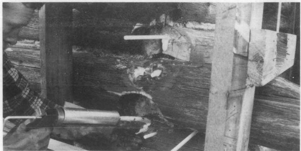
Figure 6. A flexible tube was stapled onto a caulking gun in order to fill the 12"-12 1/2" deep holes that had been drilled into the sound end of the historic log. The individual hole was filled two-thirds with epoxy adhesive and a 1/2" diameter fiberglass reinforcing rebar was then inserted. Photo: Harrison Goodall.
