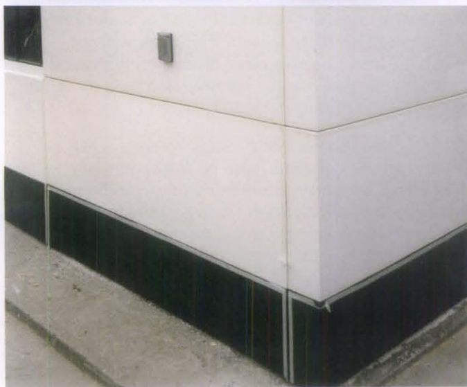
Figure 11. The porcelain enamel facade of this former Texaco station (1960) had numerous dents and scratches that had exposed the steel beneath the enamel to deterioration (top). Rehabilitation work included repairing localized damage to the panels and blending patched areas to match adjacent historic material, replacing sleepers beneath the panels (center), replacing severely damaged panels with like material, and recaulking the joints (bottom). Photos: John Vaughan, Architectural Conservation Services.
