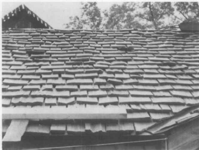
15. These commercially available roofing products with rustic split faces are not appropriate for historic preservation projects. In addition to the inaccurate appearance, the irregular surfaces and often wide spaces between shingles will allow wind-driven moisture to penetrate up and under them. The excessively wide boards will tend to cup, curl and crack. Moss, lichens and debris will have a tendency to collect on these irregular surfaces, further deteriorating the roofing. Photo: Sharon C. Park.
