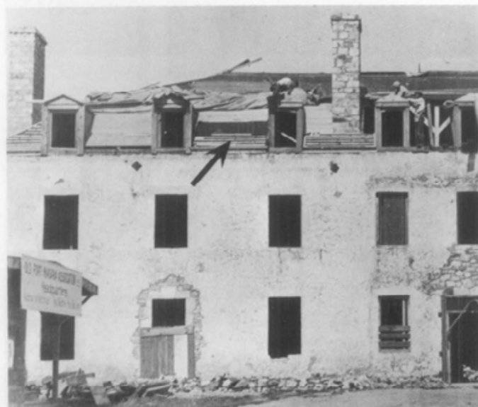
9. This 1927 view of the resingling of the French Castle at Old Fort Niagara, N.Y., shows the wooden sleepers being laid (see arrow) over solid sheathing in order to raise the shingles up slightly to allow under-shingle ventilation. Note that the horizontal strips are not continuous to allow airflow and trapped moisture to drain away. This cedar roof has lasted for over 60 years in a harsh moist environment. Photo: Old Fort Niagara, Assoc. Inc.
