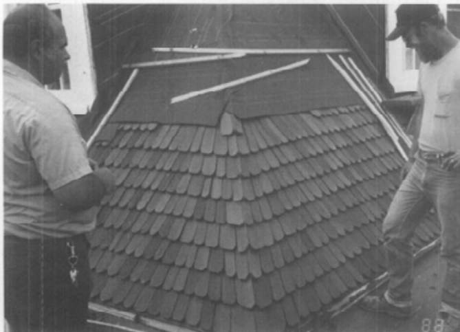
D. The fanned hips (seen here), swept valleys, and projecting ridge combs were installed as part of the re-roofing project. Special features, when documented, should be reproduced when re-shingling historic roofs.
