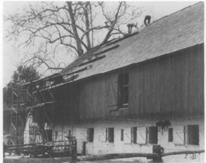
11. The replacement sawn red cedar shingles matched the deteriorated shingles exactly for this barn re-roofing. The old shingles, seen to the far left, were removed as the new shingles were installed. Even the horizontal coursing matched because the exposure length for both old and new shingles was the same. Photo: Williamsport Preservation Training Center.
