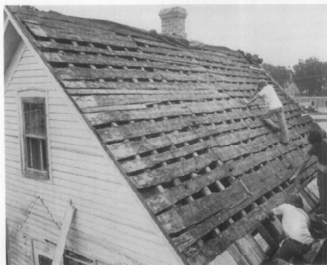
7. The resingling of the circa 1856 Stovewood House in Decorah, Iowa, revealed the original open sheathing boards and pole rafters. Sawn cedar shingles were used as a replacement for the historic cedar shingles seen still in place at the ridge. A new starter course is being laid at the eaves. Photo: Norwegian-American Museum, Decorah, Iowa.
