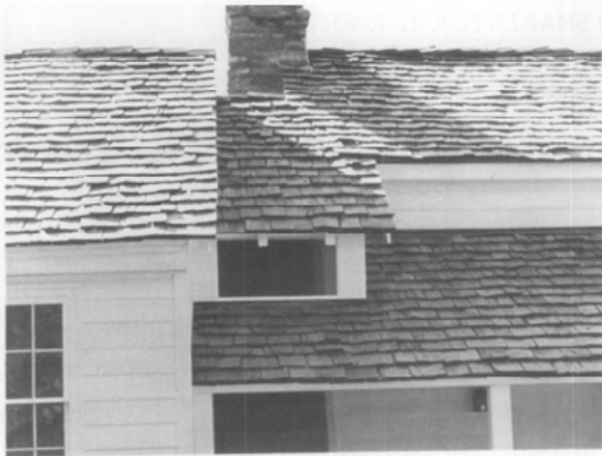
12. Inappropriately selected and installed wooden shingles can drastically alter the historic character of a building. This tavern historically was roofed with handsplit and dressed shingles of a relatively smooth appearance. In this case, a commercially available shake was used to effect a "rustic" appearance. Photo: National Park Service.
