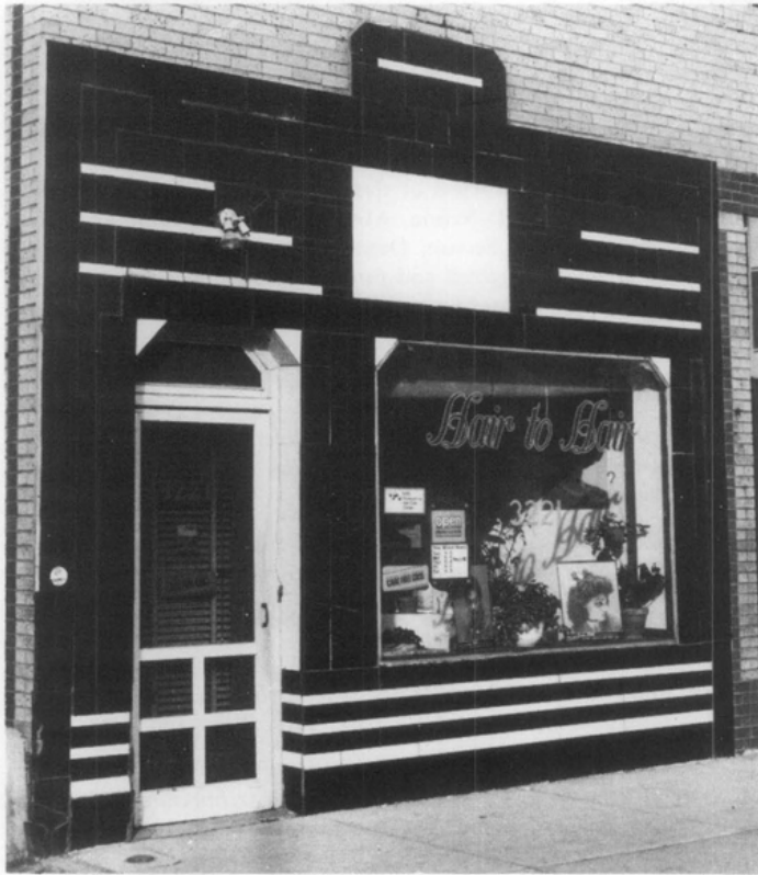
Fig. 15. Owners of this small barber shop, Denver, Colorado, have successfully preserved the historic character of their pigmented structural glass storefront by patching the cracked panels with a dark caulking compound. Photo: Gregory D. Kendrick.
