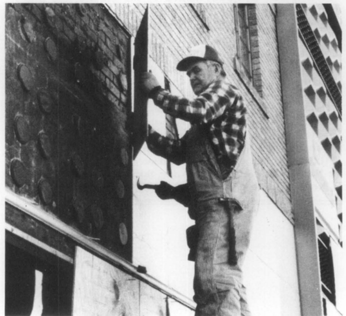
Fig. 16. A worker carefully removes a large glass panel by placing a small piece of wood between a flat prying bar and the glass, then exerting steady pressure. The majority of panels were removed without damage using this procedure. Photo: Thomas Keohan.
