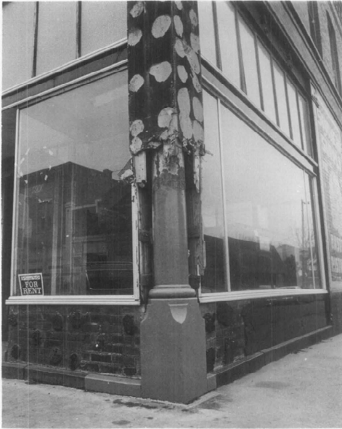
Figure 6. Storefronts of the 1940's, 50's, and 60's were frequently installed by attaching studs or a metal grid over an early front and applying new covering materials. If the existing storefront is a relatively recent addition with little or no architectural merit, begin by removing the covering materials in several places as was done here. If this preliminary investigation reveals evidence of an earlier front, such as this cast-iron column, carefully remove the later materials to assess the overall condition of the historic storefront. The black mastic visible on the lower masonry panels was used for installing pigmented structural glass. Some attachment methods for modern facings, such as mastic or metal lath, may have seriously damaged the original fabric of the building, and this must be taken into account in the rehabilitation process. Photo: Bob Dunn
