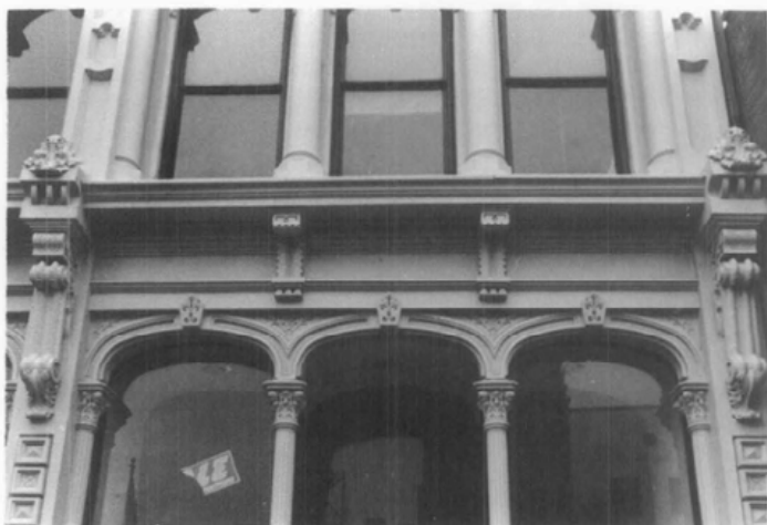
Figure 8. When the Grand Opera House in Wilmington, Delaware, was rehabilitated, missing cast-iron columns were cast of aluminum to match the original; in this particular case, because these columns do not carry great loads, aluminum proved to be successful substitute. Photo: John G. Waite
