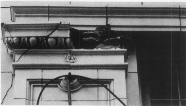
Figure 10. Structural Cracking. Structural cracking, whether static (nonmoving) or dynamic (moving or active), should be caulked to prevent water entry into the glazed architectural terra-cotta system. Note the exposed webbing.
