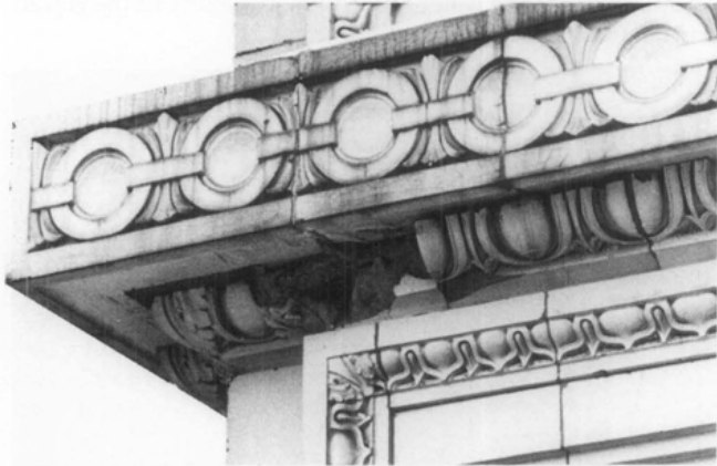
Figure 7. Material Spalling. Excessive expansion of the porous tile body caused by water and freezing temperatures produces major material spalling, a situation often difficult to repair.
