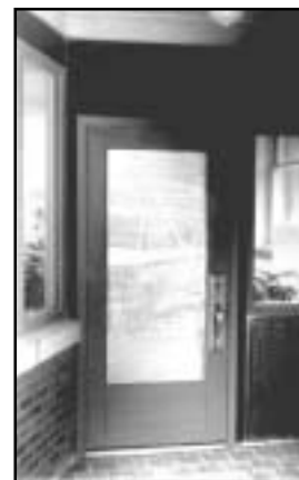
Appropriate replacement door.
