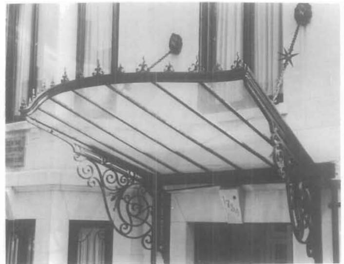
Figure 56. Wrought-iron and Glass Canopy, 1734 N Street, NW, Washington, D.C., ca. 1885. Iron is found in a variety of forms from strap hinges to fragile glass and iron combinations—such as the canopy protecting the entrance of this elegant townhouse. Glass panels were set in an iron frame with fleurs de lis on the front edge and flourishes as supporting brackets. (David W. Look)
