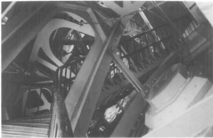
Figure 74. Stairs between the Inner and Outer Domes, U.S. Capitol, 1856–1865; Thomas U. Walter, Architect of the Capitol; Montgomery C. Meigs, engineer. The double shell dome construction is supported by 36 radiating, arched trusses. In this view of the stairs to the lantern, every element is cast iron except the wrought-iron tie rods and bolts. To the right is the back side of one of the cast-iron coffers of the inner dome. The center of the coffer can be unbolted for inspection and maintenance of the inner dome. (David W. Look)
