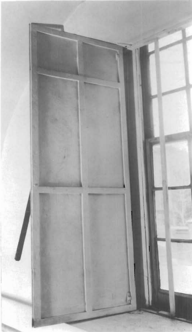
Figure 54. Wrought-iron Shutters, Arch Street Meeting House, 302-338 Arch Street, Philadelphia, Pennsylvania, 1803-1804; Owen Biddle, architect and master builder. The shutter is on the window of the "fireproof" vault used to store records. The iron shutter has a frame of hand-forged rectangular bars to which a series of rolled sheets was riveted. (George Eisenman)
