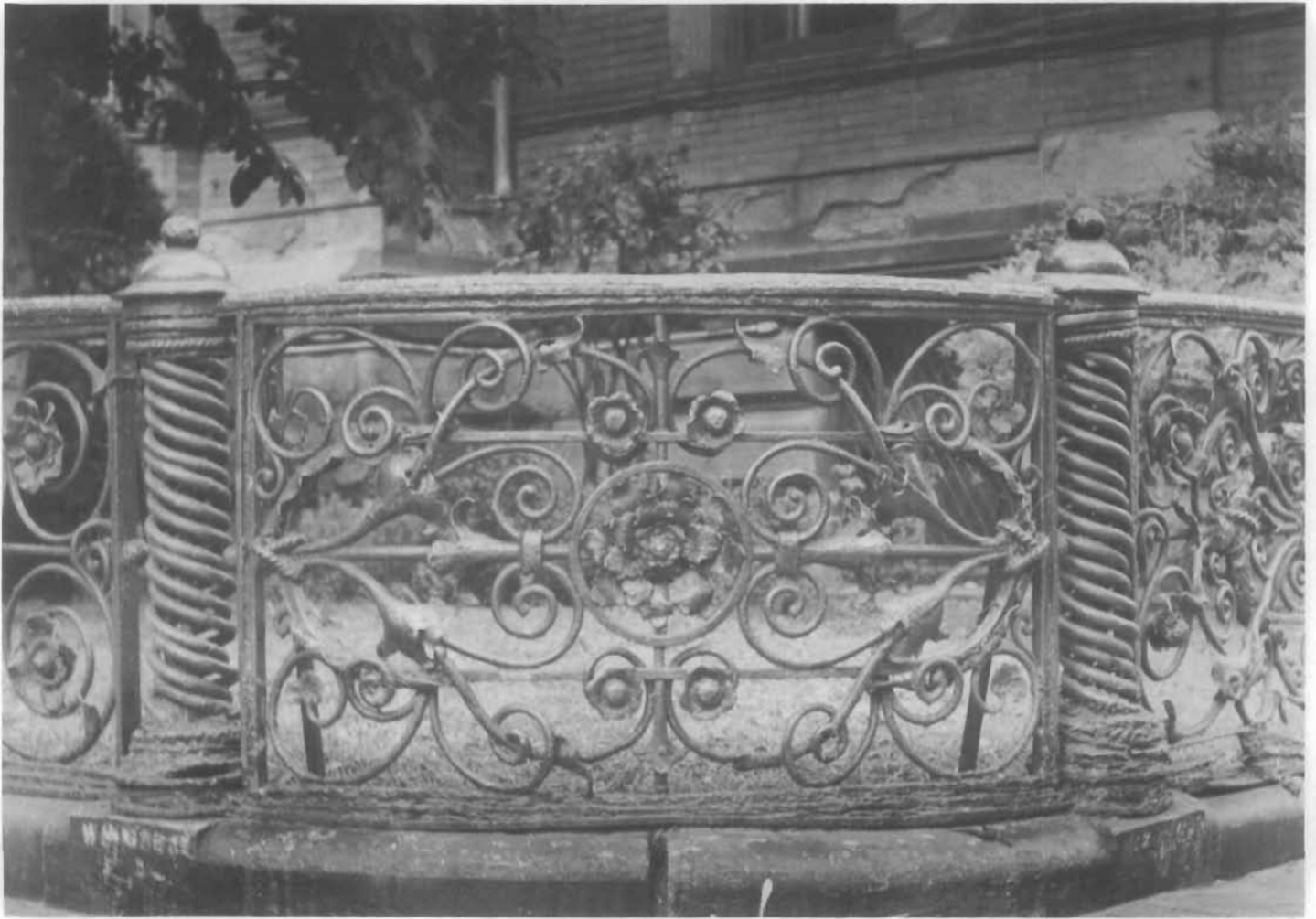
Figure 53. Wrought-iron Fence, Frederick Ames Mansion, 306 Dartmouth, Boston, Massachusetts, 1872; John Sturgis, architect. This fence was fabricated by hand from iron bars; square and round sections were hot-worked into spirals, circles, and scrolls. Even the fence posts are compact spirals of strong rods shaped about a central support to make them rigid. (Esther Mipaas)
