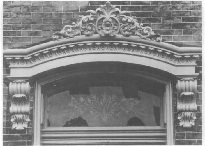
Figure 84. Cast-iron Lintel, Ben Whitmire House, 109 Jackson Street, Trenton, New Jersey, 1872. The scrollwork of the foliated lintel is clearly of cast metal; execution of such a design in stone would be almost impossible. This house also has window lintels and sills of iron, all of which were probably cast at Bottom and Tiffany's Foundry in Trenton. They were often painted stone colors with sand added for the correct texture. Residences, commercial buildings, institutions, and even industrial buildings incorporated ornate lintels and sills in their design. (Ben Whitmire)
