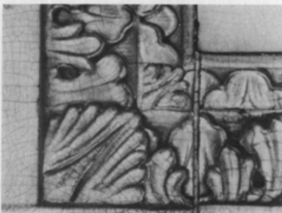
Crazing of glazed terra cotta. Photograph: National Park Service.
