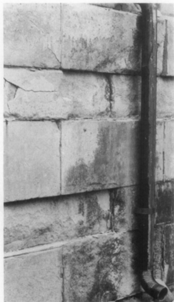
Crumbling limestone resulting primarily from excess moisture penetration. Photograph: National Park Service.
