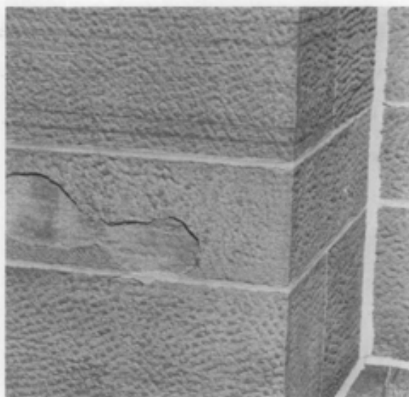
Blistering of sandstone. Photograph: Anne E. Grimmer.
