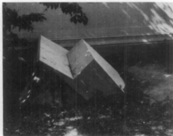
Section of marble lying on the ground at base of building after it had separated from pediment above. Photograph: Walter Smalling.
