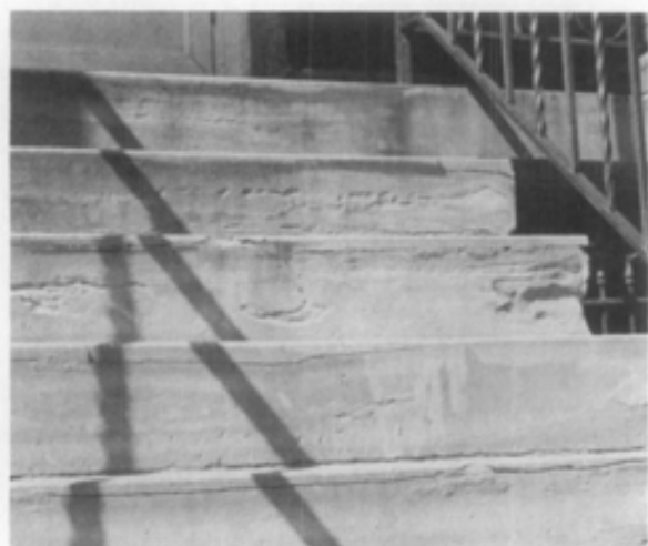
Differential erosion of sandstone steps follows bedding planes of greater and lesser resistance. Photograph: Anne E. Grimmer.
