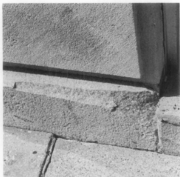
Chipping of granite sill. Photograph: Anne E. Grimmer.
