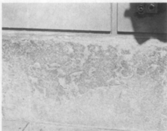
Salt fretting on granite base probably resulting from use of de-icing salts on sidewalk. Photograph: Anne E. Grimmer.
