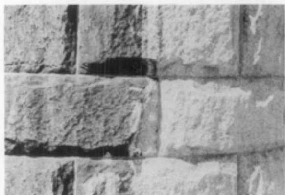
Chemical cleaning to remove urban dirt and pollution from granite without causing damage or abrasion to the surface of the stone.
