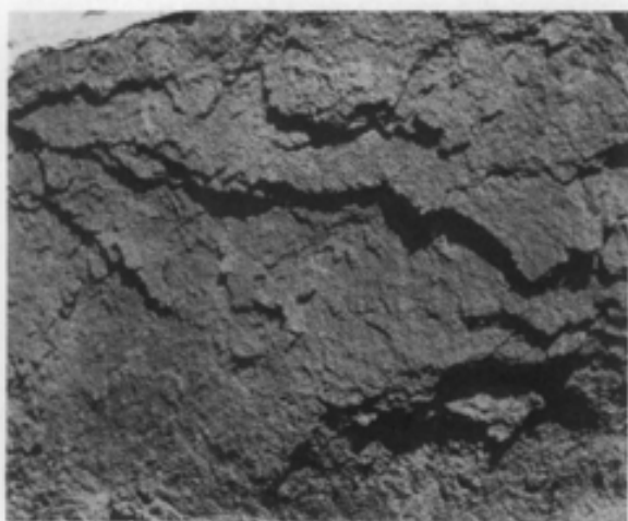
Exfoliation of sandstone. Photograph: Anne E. Grimmer.
