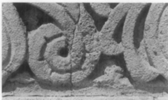
Cracking of limestone. Photograph: John H. Myers.
