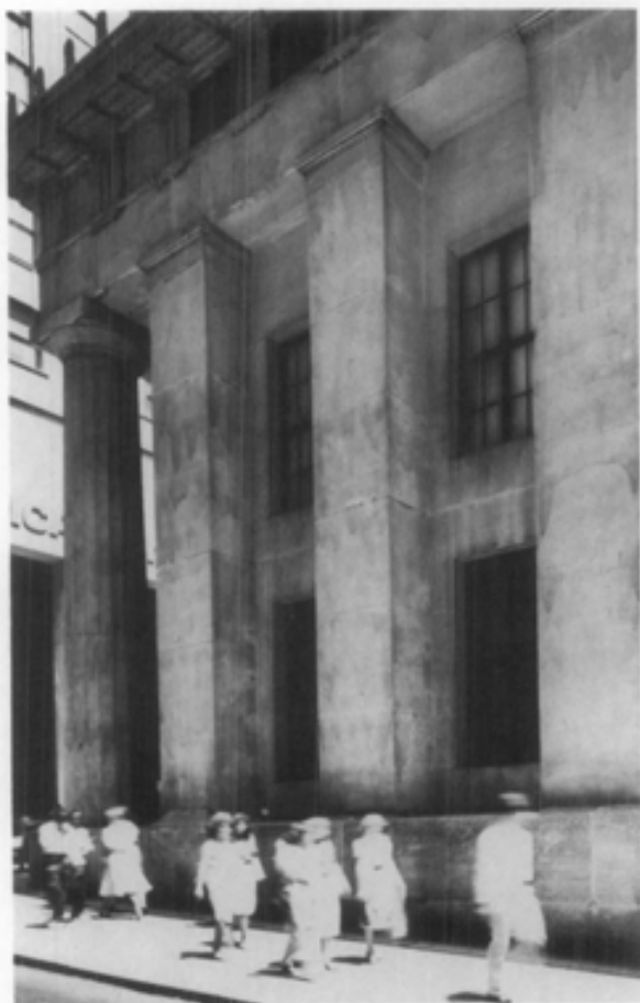
Water-repellent coating improperly applied gives a blotchy appearance to the stonework. Photograph: Walter Smalling.
