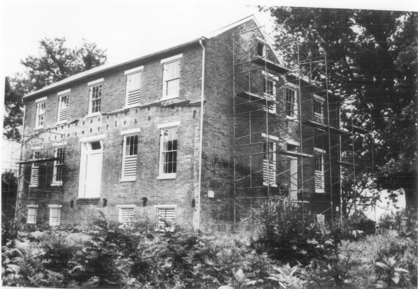
Figure 6. The window louvers installed in the Worthington House have proven effective over the past two years in providing the necessary ventilation for the building. Photo: Tom Vitanza.
