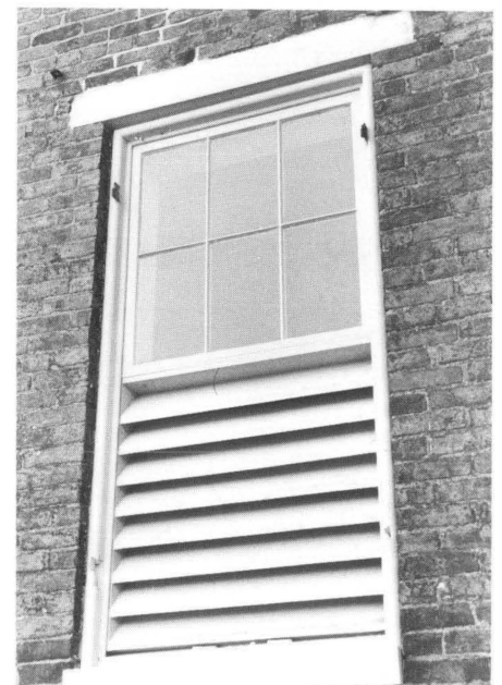
Figure 3. The exposed edges of the louver slats were plumb cut in order to create a water drip on the exterior. For aesthetic reasons, the louvers were painted the same color as the sash and trim. Photo: Charles Fisher
