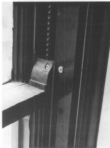
Figure 4. The only modification made to the windows was the addition of a screw through the decorative end of the sash stile to fix closed the operable portions. This decision grew out of the recommendations by the mechanical engineers. Photo: Charles E. Fisher
