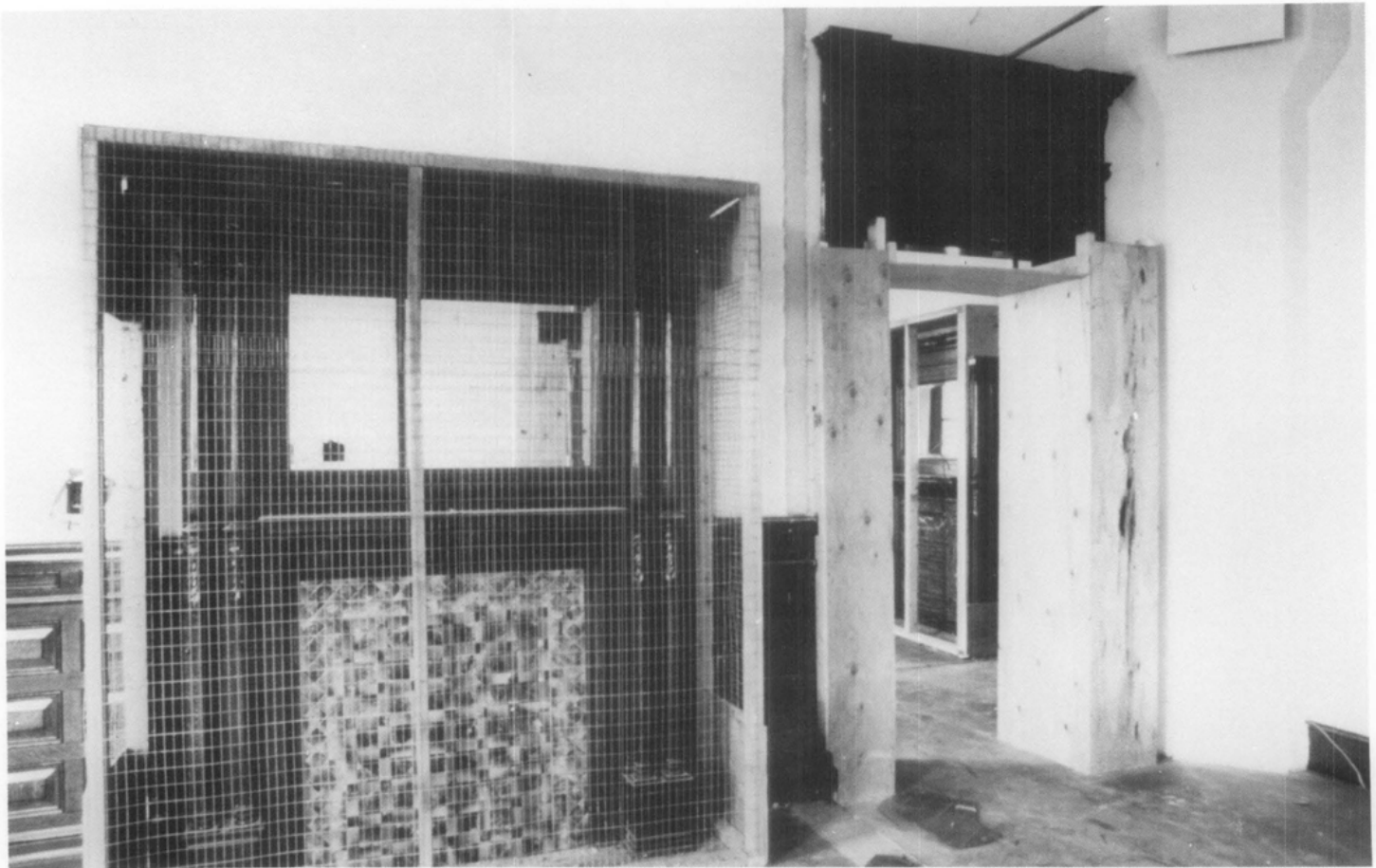
Figure 6. A self-supporting impact cage utilizing wood and wire mesh protects the fireplace. In this project, the long construction process required bidders to have visible access to features such as the fireplace. The wire mesh also facilitated monitoring during the lengthy construction. Photo and drawing: Ford Farewell Mills and Gatsch Architects.
