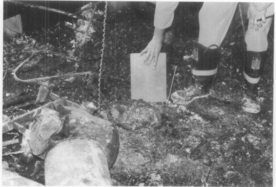
Figure 1. The spontaneous combustion of cloth rags that had been used in applying a common finishing wax caused over $1 million damage to a historic government office building in 1991. Remains of the trash can where the rags had been stored overnight is indicated by the fireman's notepad. After the cause of the fire was determined, a standard specification provision was developed for future contracts requiring the contractor to remove all material contaminated with finishing products from the site at the end of the day.
