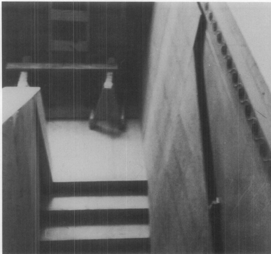
Figure 6. The balustrade on the left side of the photograph has been entirely encased in plywood to protect it from damage. Note that the kick-out at the end is due to the protrusion of the newel post. Photo: Charles Fisher.
