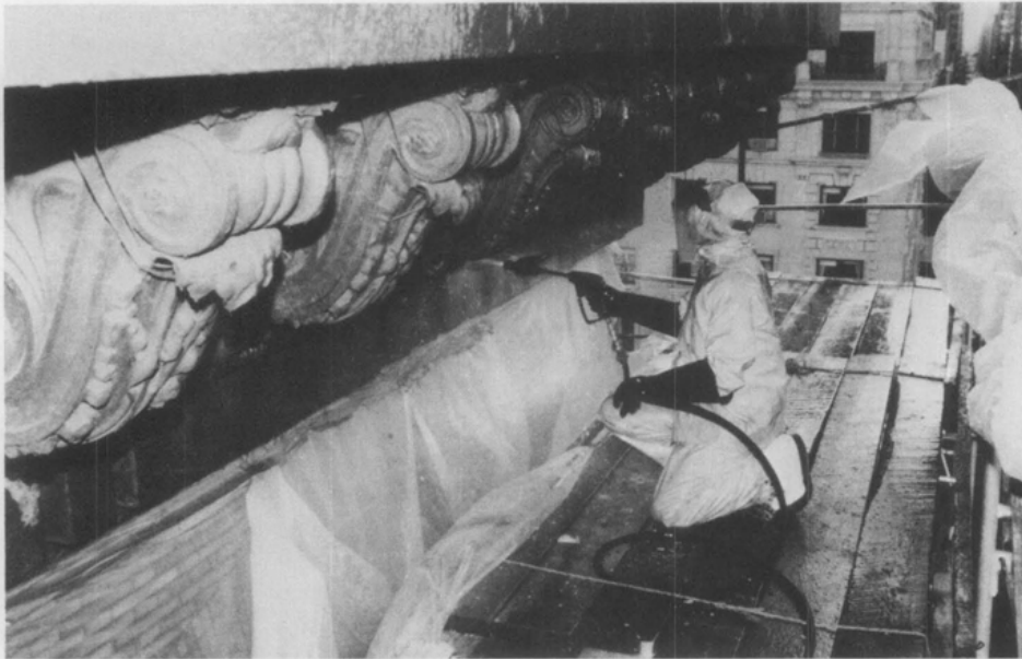
Figure 7. A water spray was used to remove most of the paint from the components of the cornice that were being retained. With the more delicate egg and dart molding, care was required to avoid possible dimpling of the metal. Steps were taken to keep water from collecting inside the cornice. Photo: Michael Devonshire.
