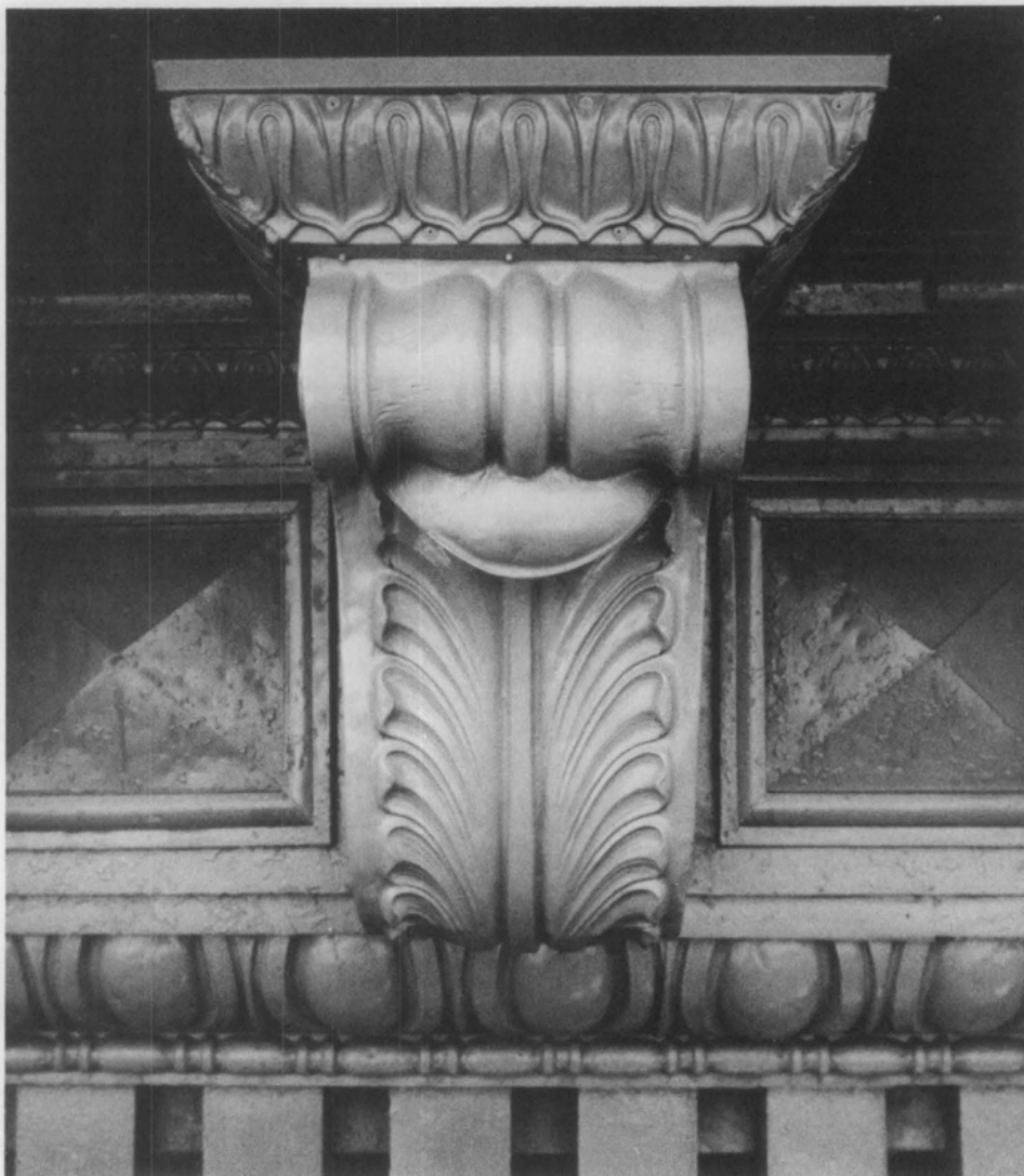
Figure 12. Detail of the completed cornice shows the new zinc modillion and the leaf and egg and dart moldings attached to the historic cornice. This repair approach, which involves in-kind replacement of deteriorated components, is the recommended treatment for such distinctive features as this cornice. Photo: Michael Devonshire.
