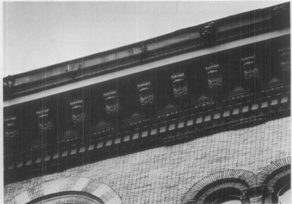
Figure 6. Three of the components of the metal cornice which required replacement because of serious deterioration are shown in this view. They are the lions' heads on the crown molding (several are missing due to failed soldered joints), modillions, and the egg and dart molding at the base of the cornice. The brake-formed galvanized steel that comprised the lineal moldings of the cornice, the soffit and dentil band were in sound condition. Photo: Richard Pieper.
