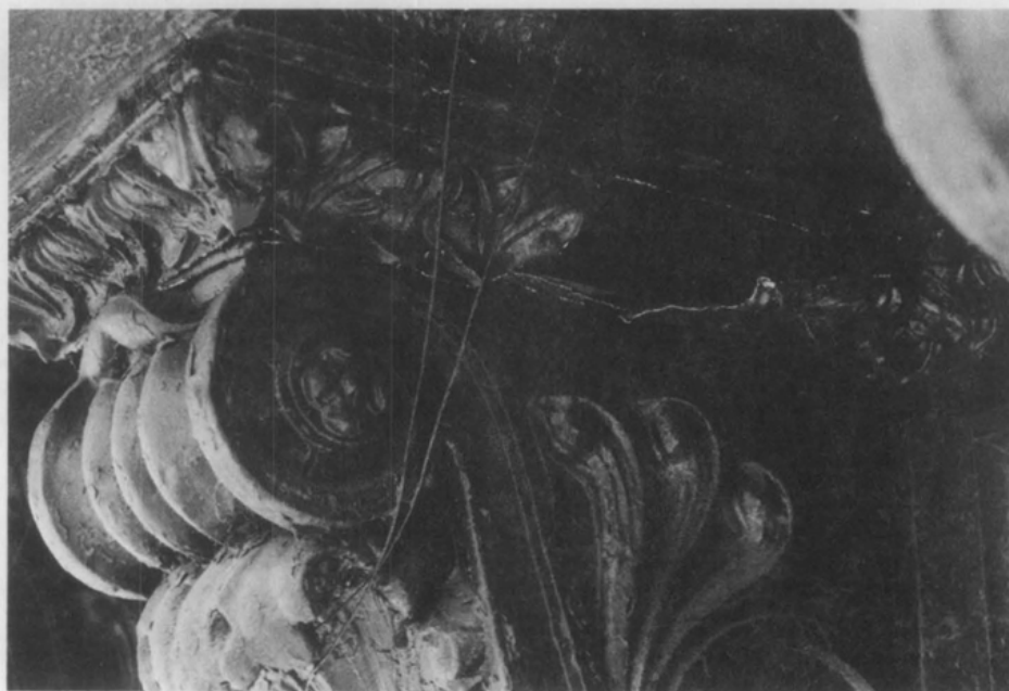
Figure 4. As shown in this view, the molding applied to the modillions was extremely deteriorated. A more serious problem was that most of the zinc modillions had fractured where the integral leaf moldings met the scrolled sides, allowing them to separate from the soffit. As a previous temporary safety measure, holes had been cut in the soffit panels to pass supporting wire beneath the modillions. Photo: Richard Pieper.
