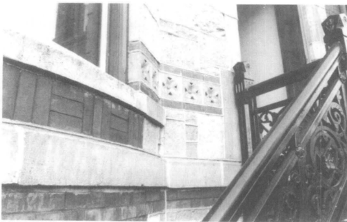
Figure 11. Close-up views of the newly installed pre-cast concrete units and the reinstated original brick. Photo: James Smith
