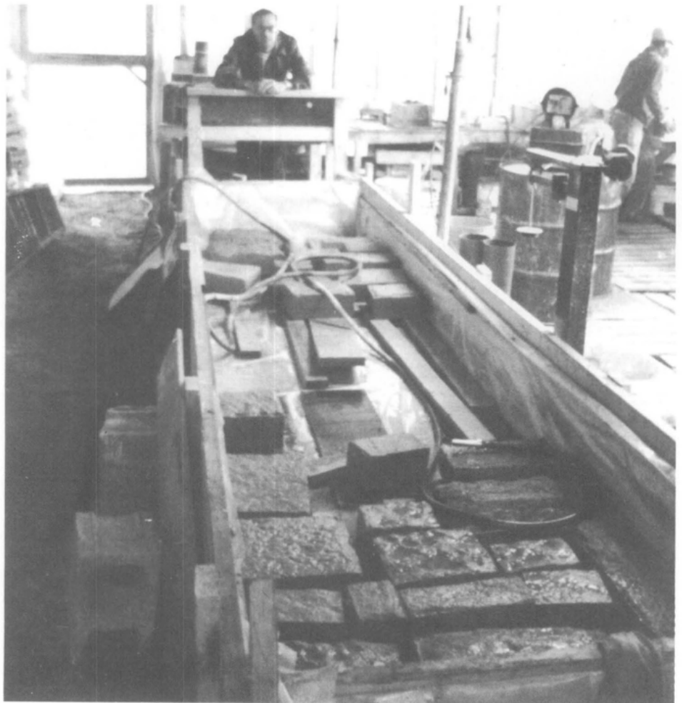
Figure 8. After soaking for 6 hours to remove soluble salts in a polyethylene-lined wood water tank, the pre-cast units were allowed to dry for another 6 hours. This process was repeated 3 times for each pre-cast unit. Photo: James Smith
