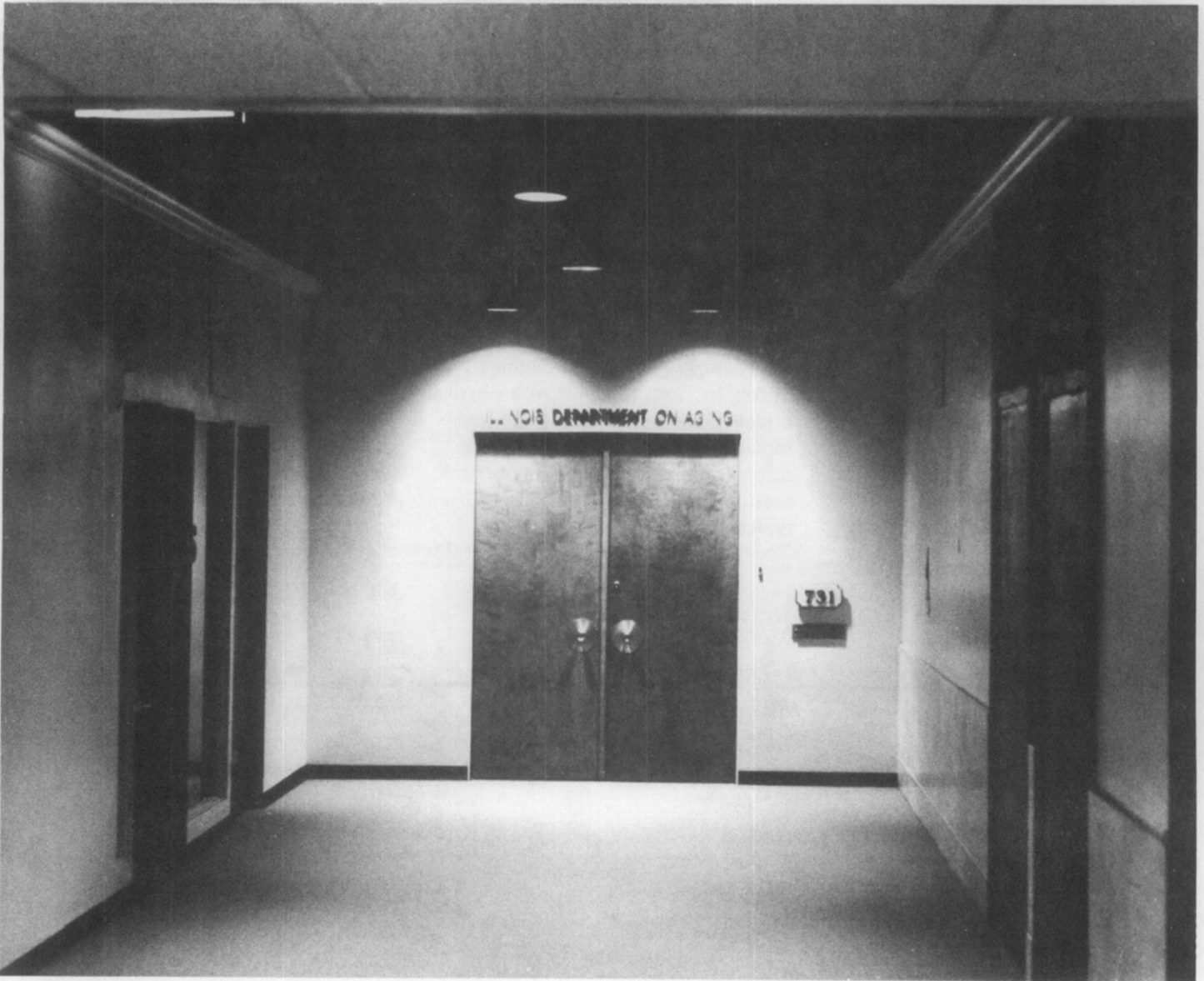
Figure 2. Typical condition of public corridors prior to rehabilitation. Glass and oak corridor partitions and much of the marble wainscot was either removed or covered. Ceilings were suspended and sections of the corridor plan were shortened or removed. Photo: William S. Donnell
