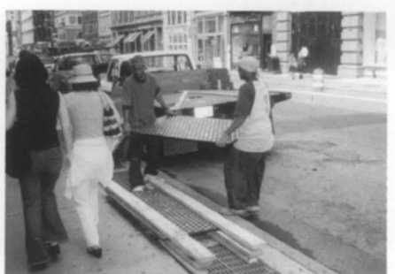
Figure 11. Just prior to installation, each panel was lifted by hand from the back of a truck and stacked on the sidewalk.
