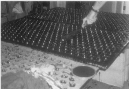
Figure 7. Cleaned and repaired panels were painted with two coats of oil-based metal primer and three alkyd gloss enamel top coats.
