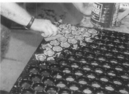
Figure 10. The grout remained water-soluble until it hardened, enabling workers to remove excess material and smooth the joint between the lens and cast-iron with a sponge.
