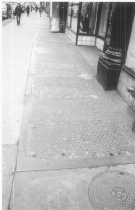
Figure 2. At the outset of the restoration project, the original cast-iron and glass vault lights in front of the building's storefront were in poor condition.
