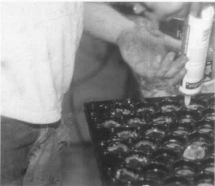
Figure 8. Before the glass lenses were set, a ring of silicone was placed along each flange on the lower edge of the opening. The silicone kept the lens centered in the cavity while a waterproof grout was used as the main sealer.
